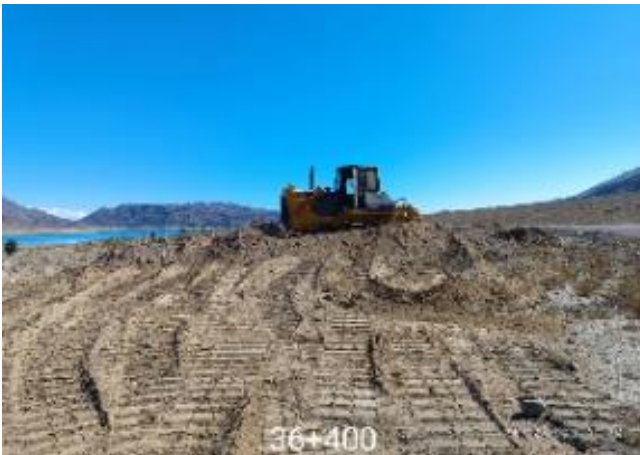
Photo 71. Unsuitable soil dump levelling at km 36+400. September
