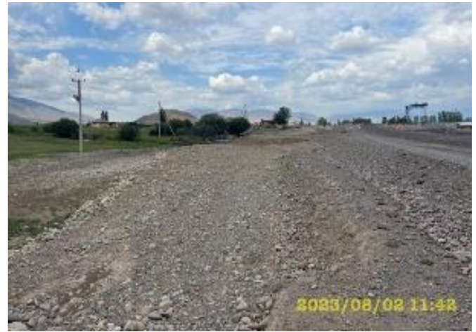
Photo 114. Site of the bypass road, after reclamation and drainage of the adjacent flooded site.
