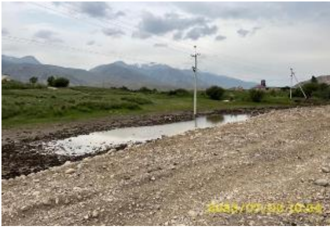
Photo 113. Bridge bypass road at km 86+261. r. Sazdyn-Suusuu River, requires reclamation and drainage of the adjacent site flooded due to bypass road construction
