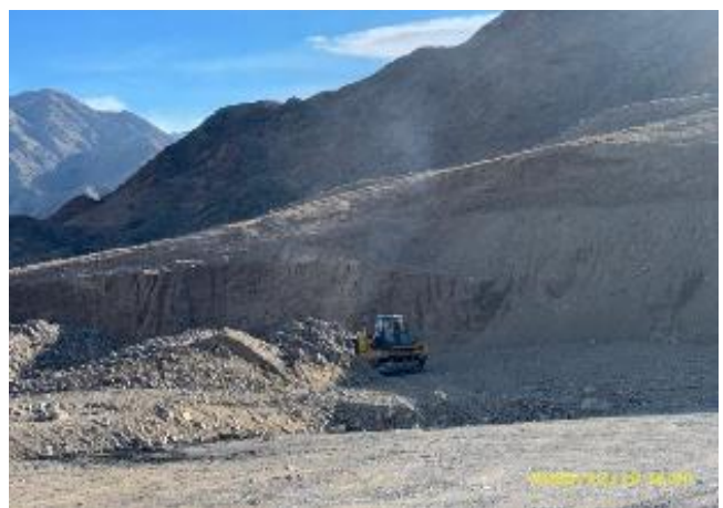
Photo 66. Quarry's technical levelling at km 34+240 and stabilizing quarry's slopes a safe condition. December
