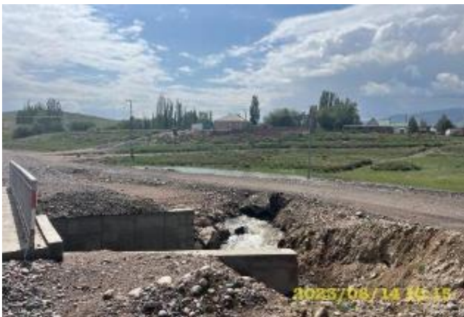
Photo 111. Bypass road of bridge at km 86+261. r. Sazdyn-Suusuu, Construction of bridge is completed, bridge access is open. The bypass road is subject to reclamation.
