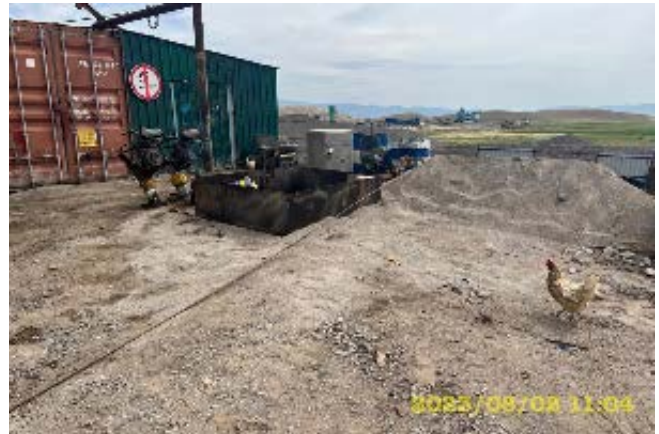
Photo 86. Lot 2. Production base, site adjacent to the oil storage warehouse after cleaning
