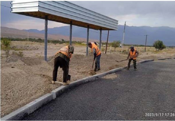
Photo 19. Earthworks on the arrangement of a bus stop in Tash-Saray village. September.
