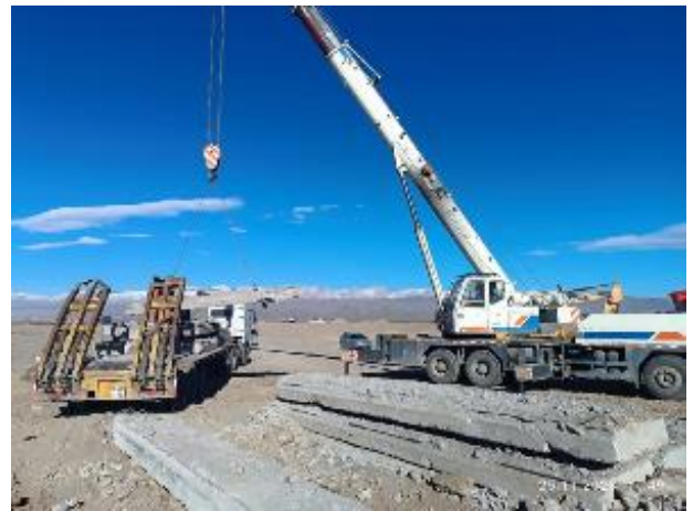
Photo 98. Dismantled parts removal of the temporary bridge of bypass road at km 62+500
