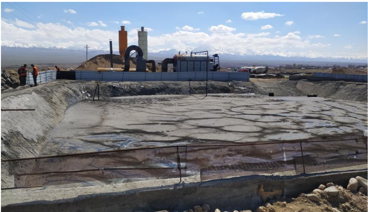
Figure 10: Bitumen pit. The bitumen pit is equipped with reinforced concrete liner and a floor to prevent the infiltration of petroleum products into the soil.
