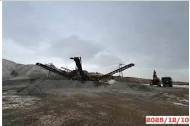
Photo 41. Production site, km 167+360 RHS, The CSP was not working.
