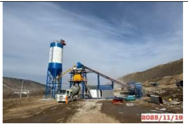
Photo 18. Production site, km 202+220 RTS, concrete production, for the construction of bitumen storage pit.
