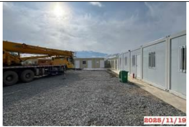
Photo 16. Production site, km 202+220 RHS, the camp territory is in satisfactory sanitary condition.
