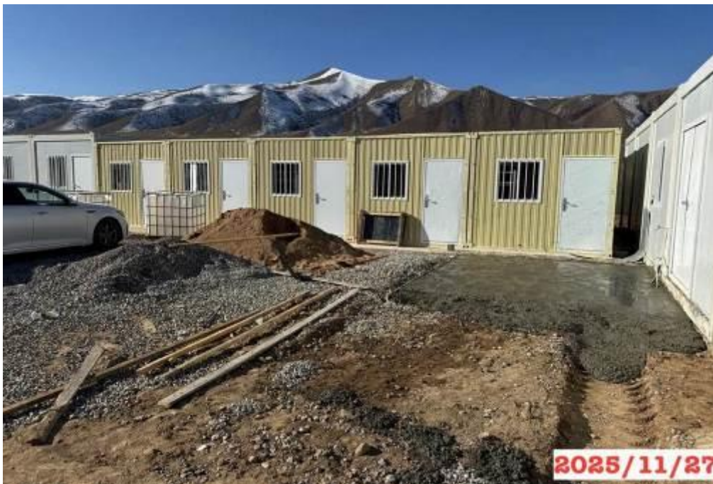
Figure 20: Chyrak Camp, km 202+220 RHS. The camp's area is being backfilled with inert material.
