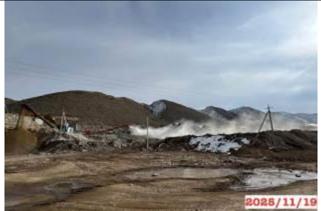
Photo 20. Production site, km 202+220 RHS: significant dust emissions are visually observed during CSP operation.
