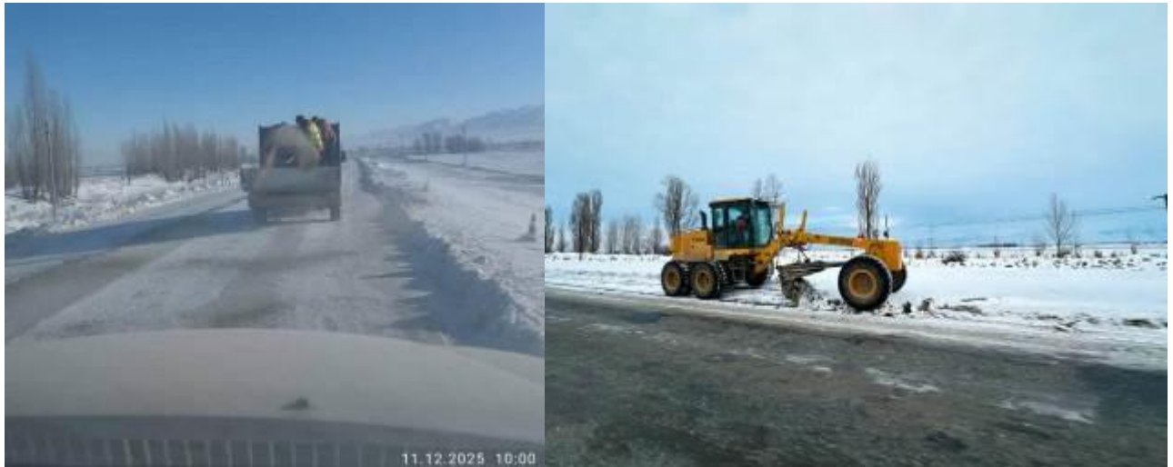
Figure 45: Clearing the road of snow and sprinkling it with inert material along the entire road section
