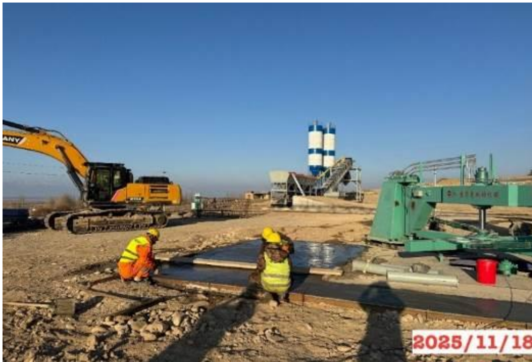
Figure 16: Production site, km 167+360 RHS, construction work on the construction of a reinforced concrete product (RCP) production facility.
