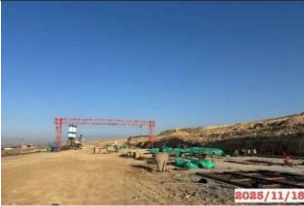
Photo 13. Production site, km 167+360 RHS. The CBP and CSP sections; the sanitary condition of the area is satisfactory.
