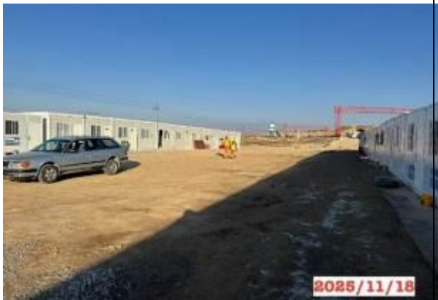
Photo 11. Production site, km 167+360 RHS, construction workers' accommodation camp. The sanitary conditions in the area are satisfactory.
