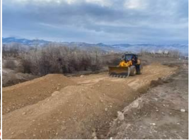
Photo 32. Lot 1. Earthworks for the construction of an embankment on the site km 153+160-153+500 RHS, 3rd layer
