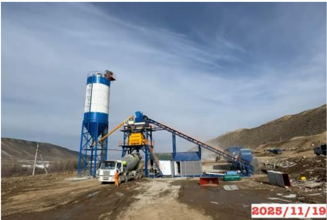
Figure 18: Production site, km 202+220 RHS, concrete production, for the construction of a bitumen storage pit.
