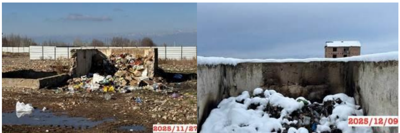
Figure 43: The Chyrak camp, km 199+460, LHS. The storage conditions for solid waste do not meet environmental and sanitary requirements
