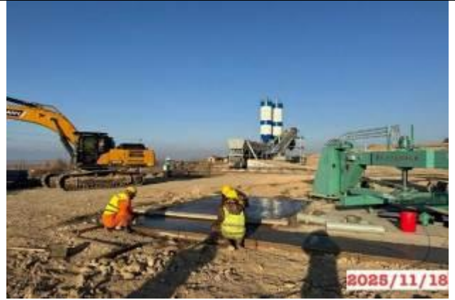
Photo 14. Production site, km 167+360 RHS, construction work on the construction of a reinforced concrete products manufacturing site.
