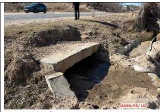
Photo 3. Debris flow passage on km.151+020 LHS. outlet
