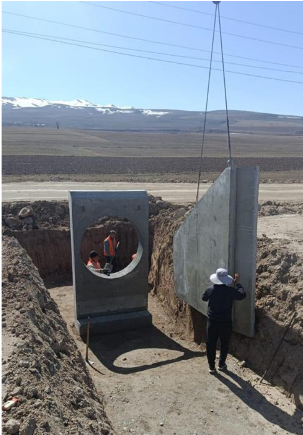
Figure 9: Installation of the headwall and wingwalls of the reinforced concrete pipe with a 1.5 m opening at km 193+995.
