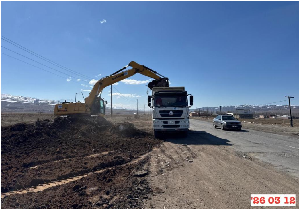
Figure 5: Clearing and grubbing of the widened section of the embankment at km 198+400 LHS.
