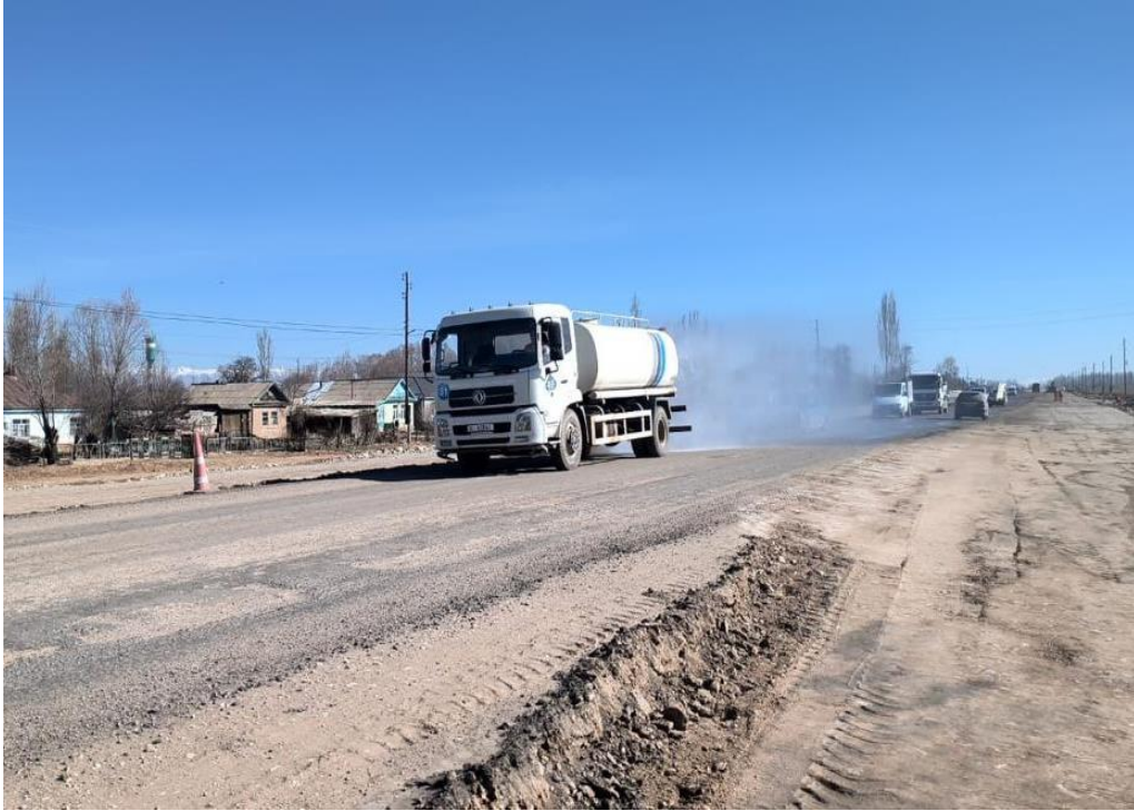
Figure 46: Suppressing dust in embankment construction areas to prevent poor visibility on the main road
