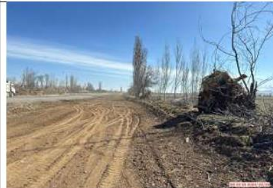
Photo 12. Km. 202+700. Big roots of cut trees, left on the edge of the road
