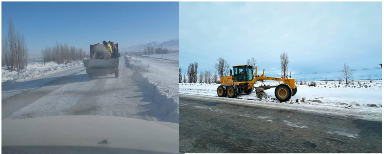
Figure 47: Clearing the road of snow and sprinkling it with inert material along the entire road section
