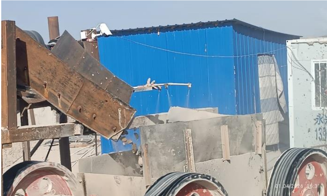
Figure 18: The irrigation system is installed in the receiving bin, as well as on the converter lines.
