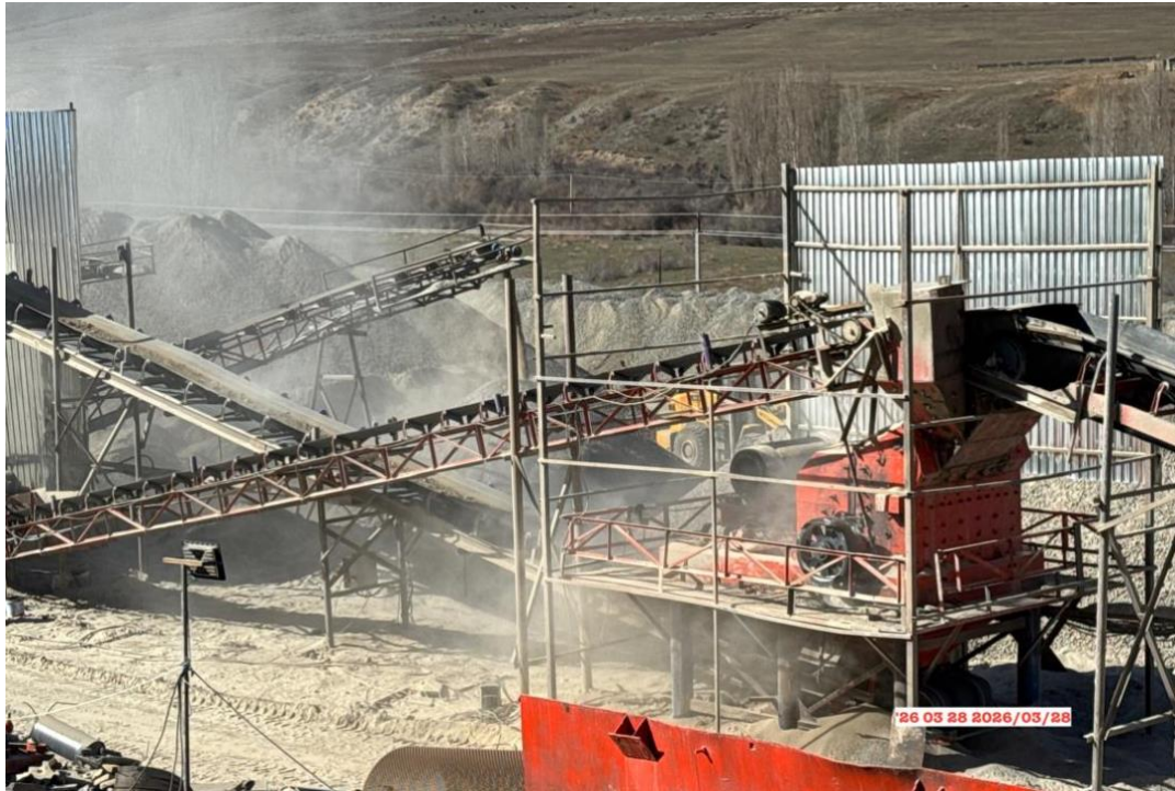
Figure 11: Production site, km 202+220 RHS, dust emission during operation of the CSP
