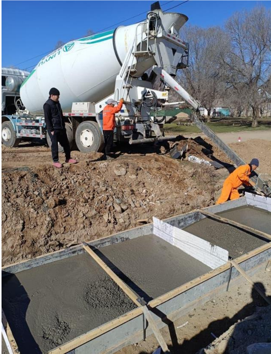
Figure 10: Concrete pouring of the foundation of the reinforced concrete pipe with a 1.5 m opening using B30 concrete at km 196+097
