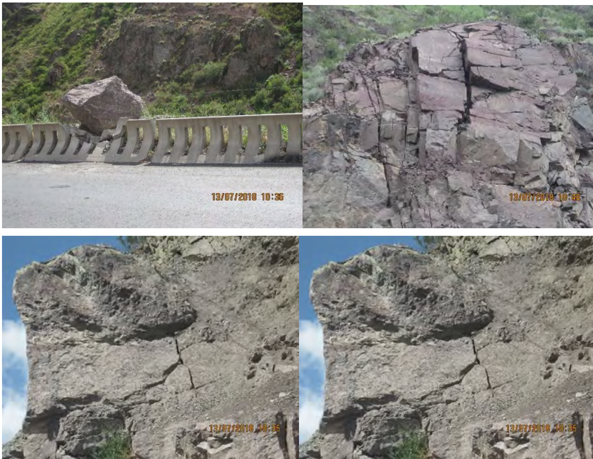
Figure 8 Danger of rockfall
