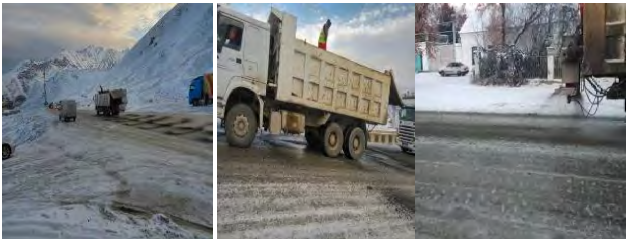
Figure 5 Clearing of road surface during the winter period - minor repair of pipes.
