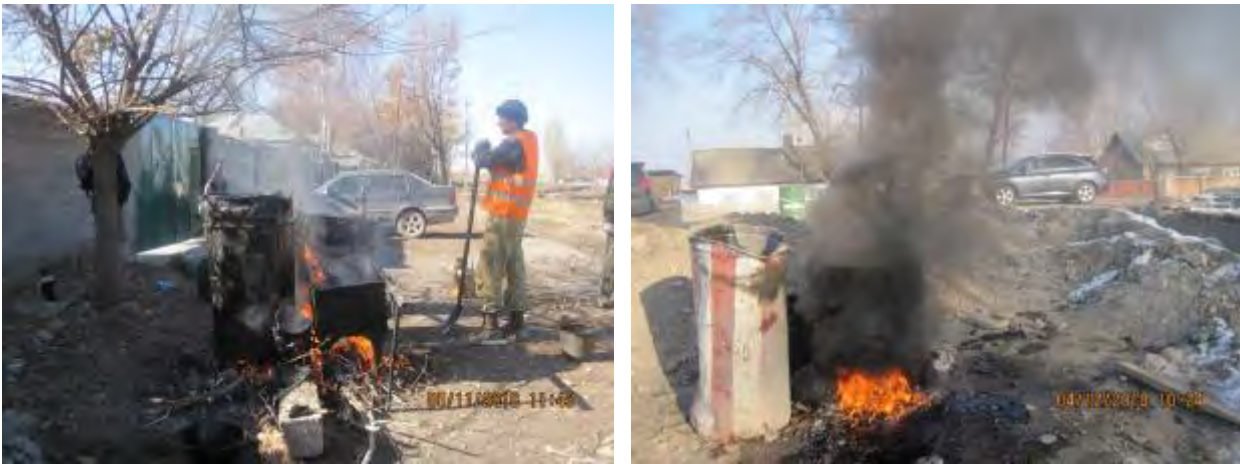
Figure 31 Violations in the melting of the bitumen during the waterproofing of culvert pipes
