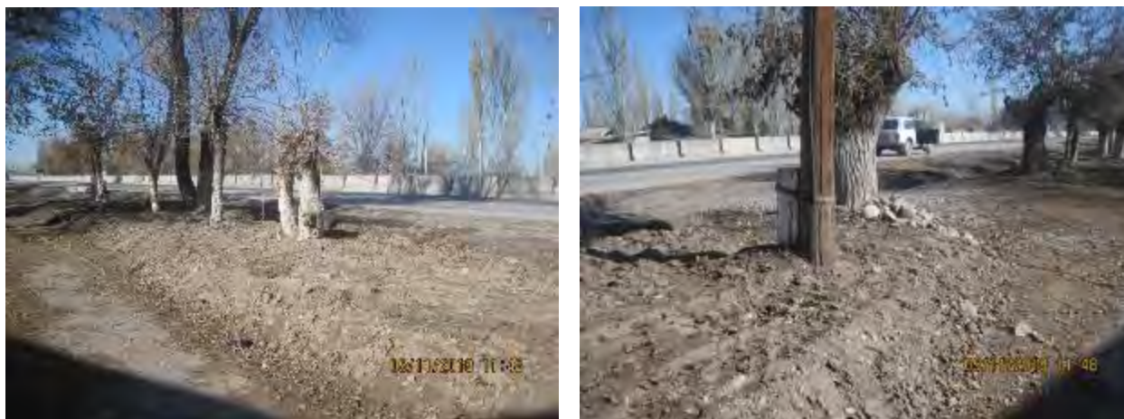
Figure 47 Stems of trees during installation of concrete culvert chutes before and after clearing of stems from the soil
