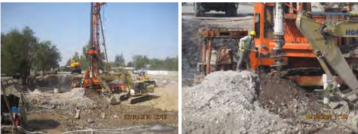
Figure 9 Construction of the bridge over Ak-Suu River on bore hole piles on the left bank
