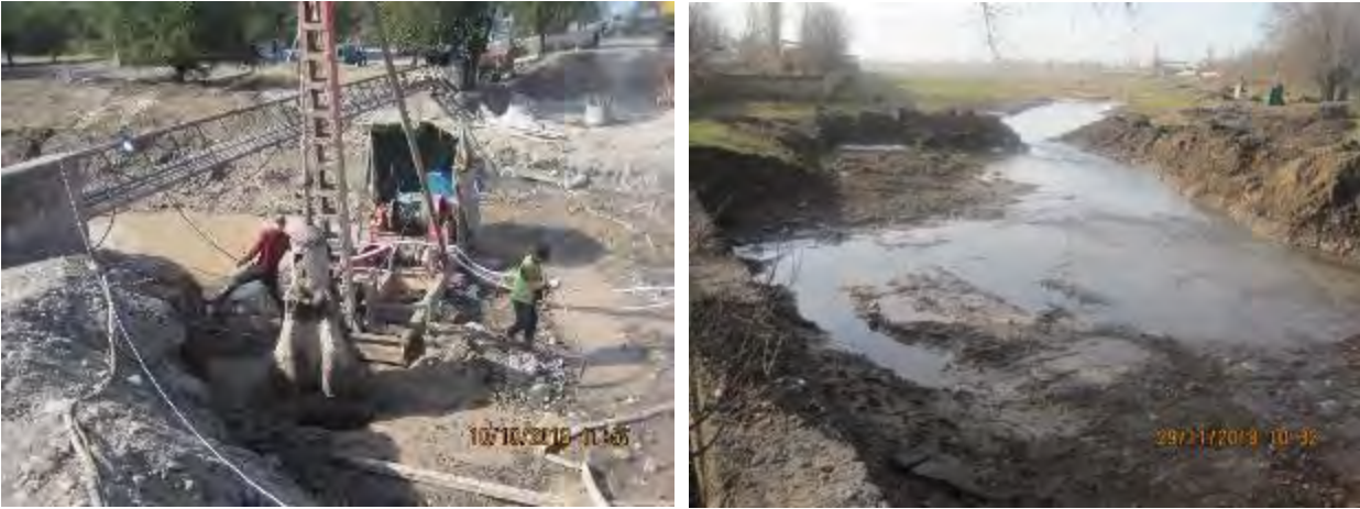
Figure 10 Construction of the bridge over Ak-Suu River on bore hole piles on the right bank
