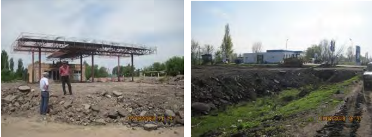
Figure 61 Taking out of old asphalt for backfilling of private areas at the request of the residents
