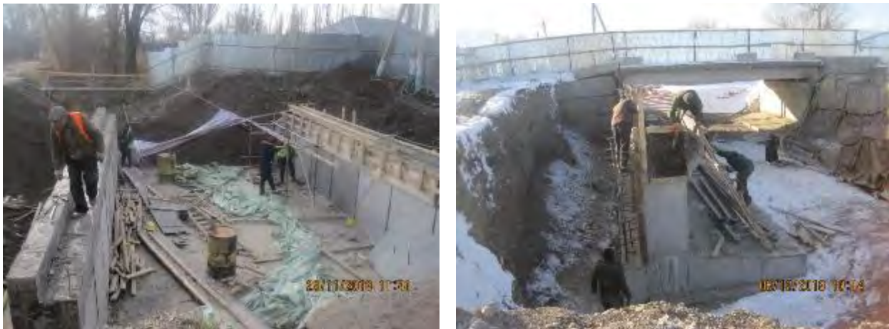
Figure 65 Carrying out of works at height without personal protective means
