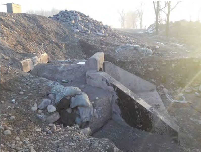
Figure 33 The pipe with an extra section
