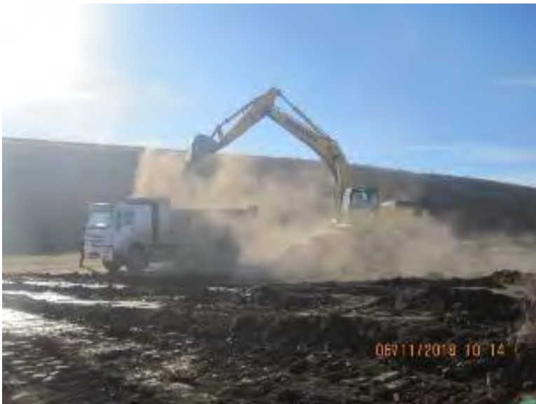
Figure 38 Dust formation during carrying out of works at the borrow-pit
