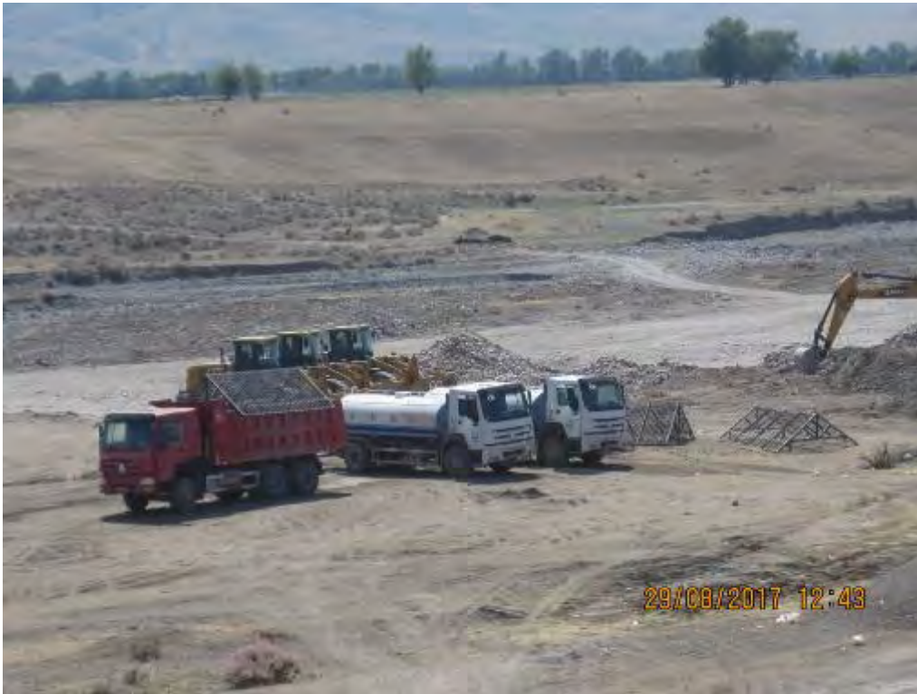
On the road from the Aksu 2 borrow pit, which leads to the village, a partitioning trench is made, so that no cars can cross it.
