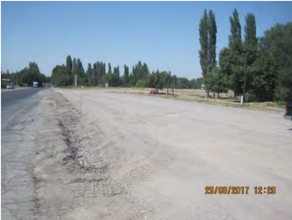
Works are also carried out on the south side of the road.
