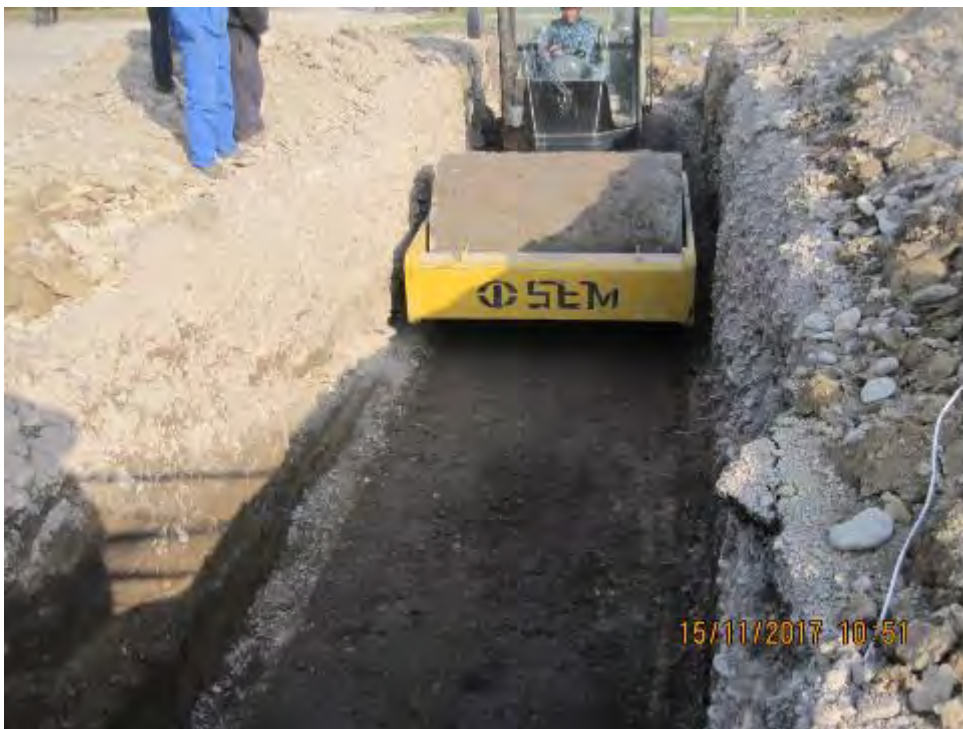
The photo shows the ramming of the base under the culvert without vibration mode
