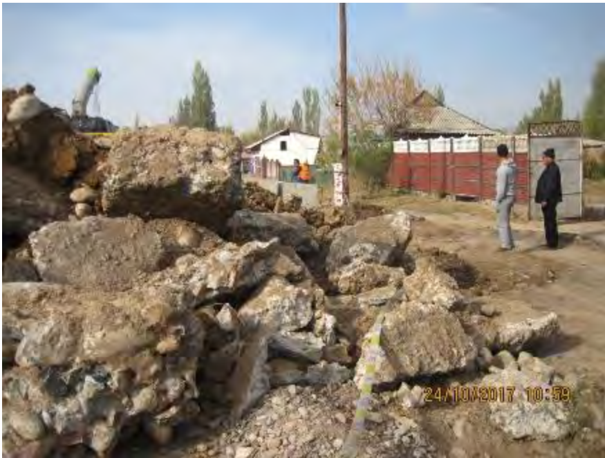
Reinforced concrete waste
