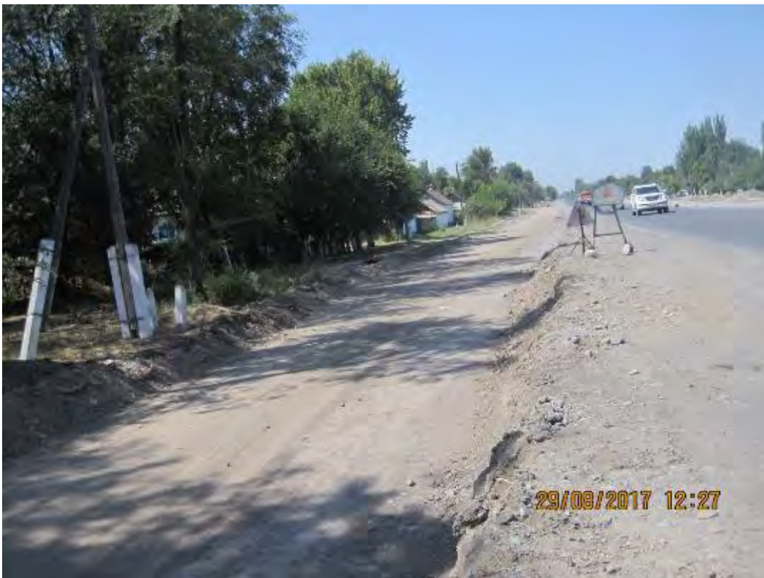
The installation of culverts continues on the north side of the road
