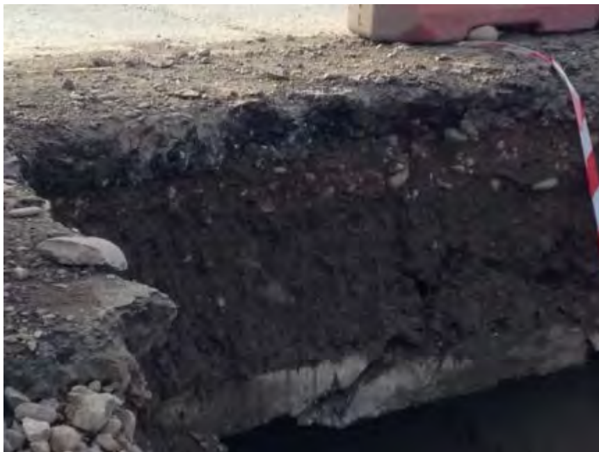
Figure 15. Work area left with undercut banks, >1m high a danger of cave in, and lower panel showing where culvert removed and road surface in imminent danger of collapse
