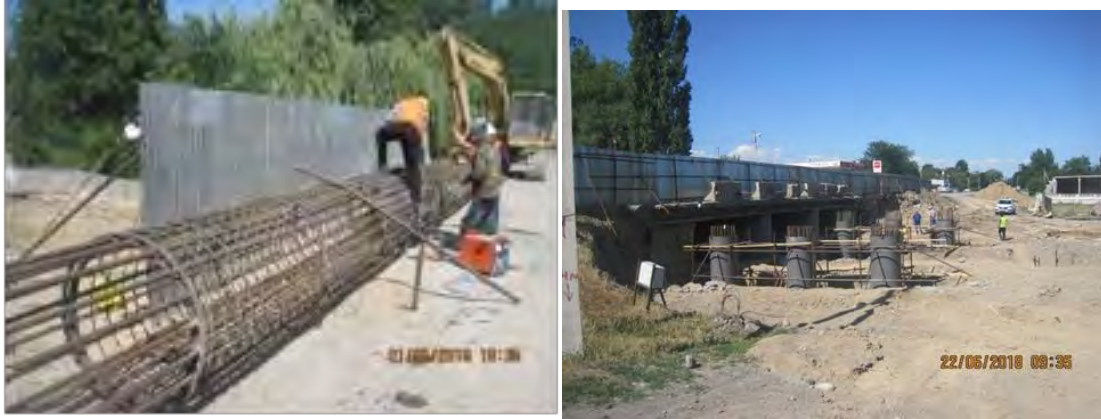
Fabrication of rebar framework for bridge piers and piers being poured-in-place in dry riverbed.
