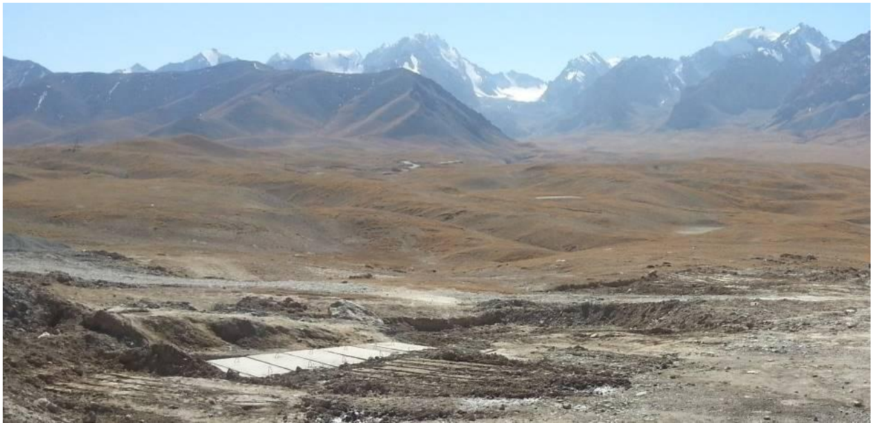
Figure 36: Septic Tank installed behind Camp – Emptied to facility at Naryn
