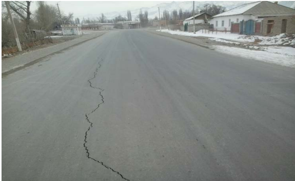
Figure 1: Frost-heave Cracks at km7+400-7+420, 22 January 2014
