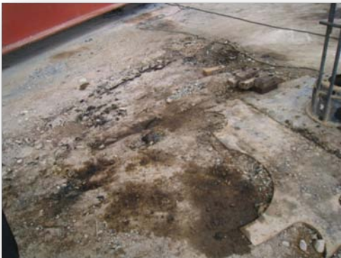
Picture 3. Team 2: Spots of oil are numerous and big
