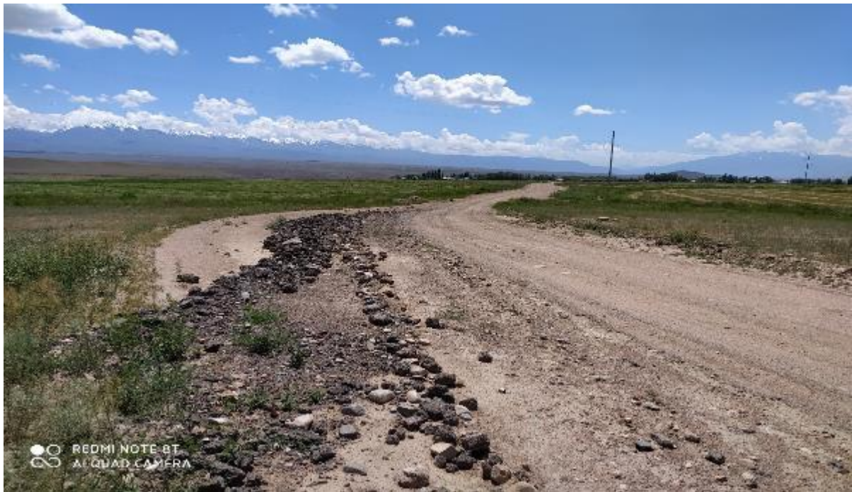
Figure 28. Leveling after backfilling with old asphalt on a country road in Epkin v.
