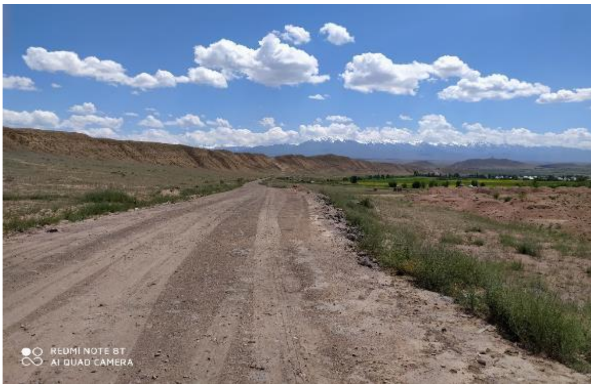
Figure 29. Removal and leveling of old asphalt in Bash-Kuugandy v. (road to the local Kara-Keche coal deposit)
