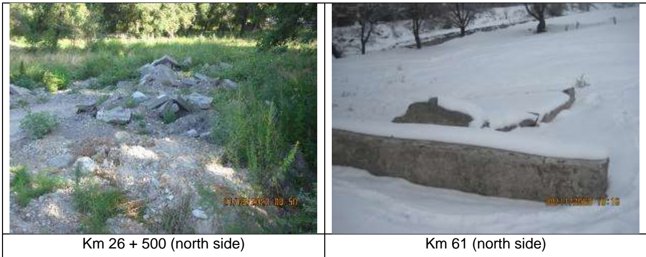
Figure 71 Reinforced concrete waste on the road
