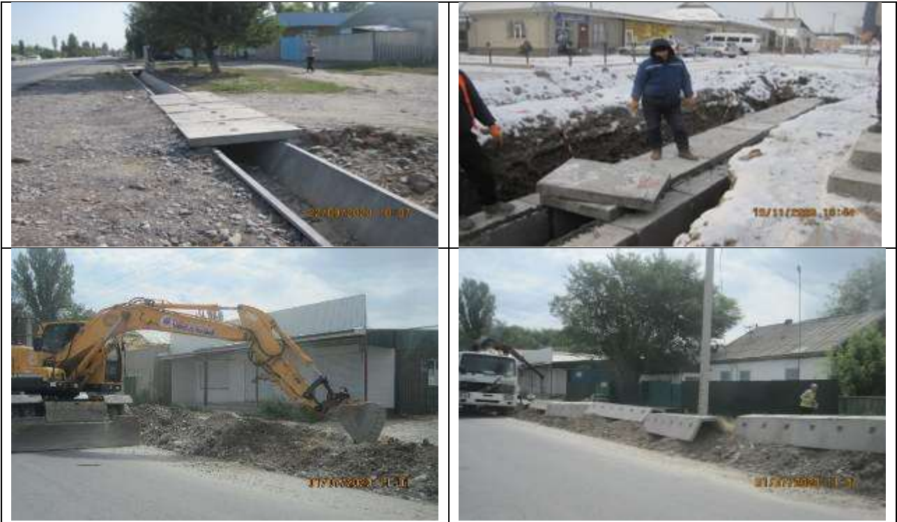
Figure 7 Construction of roadside culvert chutes and junctions at the streets adjacent to the road
