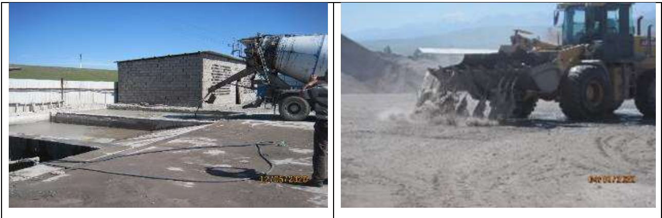
Figure 45 Washing of concrete mixers. Watering the territory of the production site with washing water
