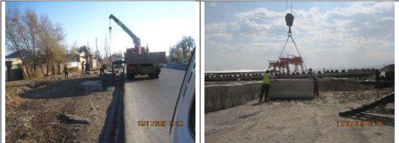
Figure 77 Violations of safety precautions when moving loads with a crane and working at height
