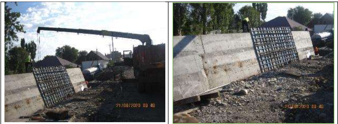
Figure 38 Violation of safety precautions during work at height
