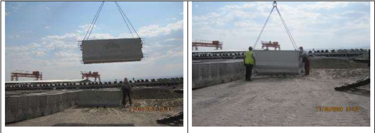
Figure 46 Violations of safety precautions when working with the crane. Lack of personal protective equipment
