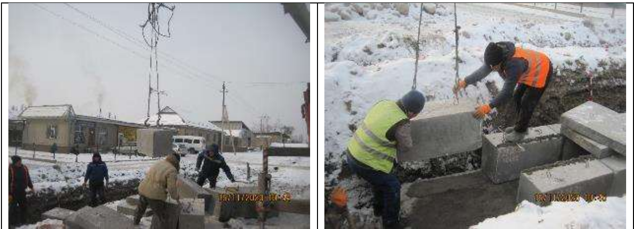
Figure 33 Violation of safety precautions during installation of culvert chutes
