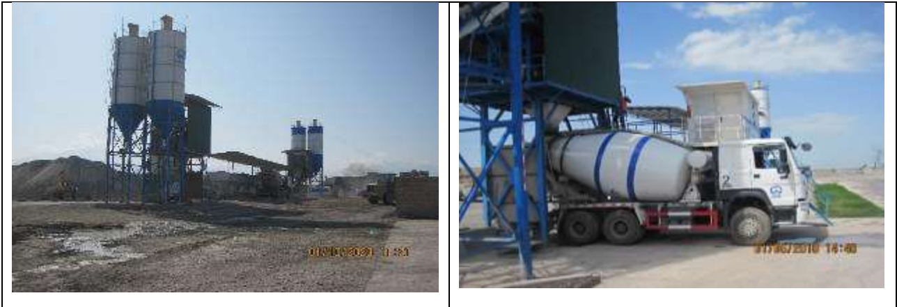
Figure 18 Concrete Mixing Plant
