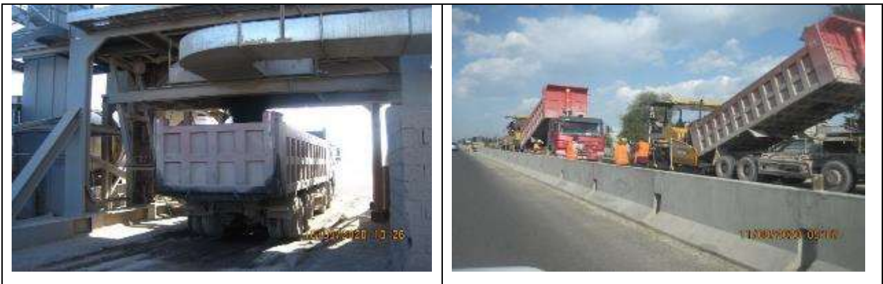
Figure 19 Loading asphalt mixture into dump trucks and unloading it into asphalt pavers
