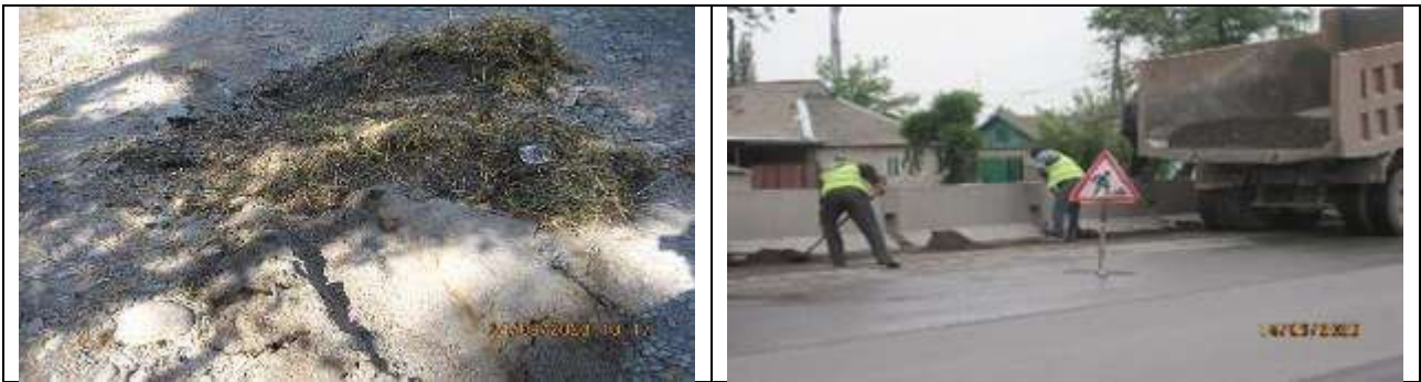
Figure 35 Asphalt and plant waste on the road shoulders formed during the strengthening of the parapet
