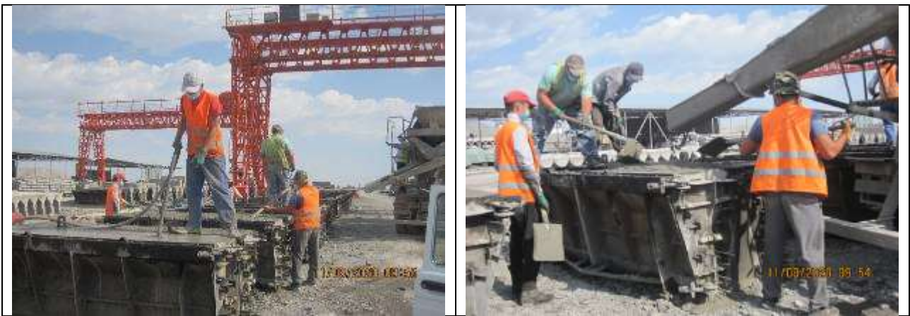
Figure 47 Lack of personal protective equipment for workers at the site for the production of reinforced concrete products when lifting and moving cargo
