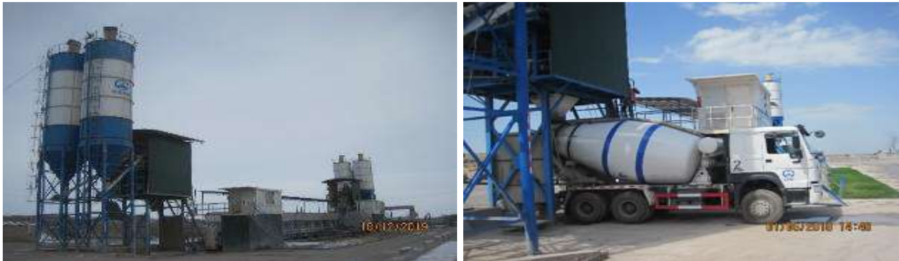
Figure 17 Concrete mixing plant
