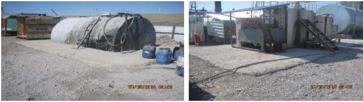
Figure 38 Impervious protective coating around the chemical storage tanks
