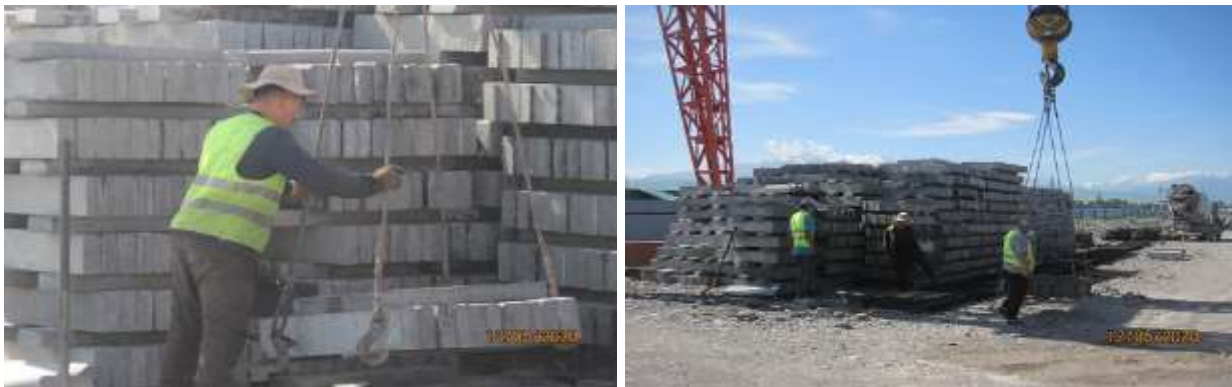
Figure 43 Lack of personal protective equipment of workers at the site of production of reinforced concrete products when lifting and moving loads
