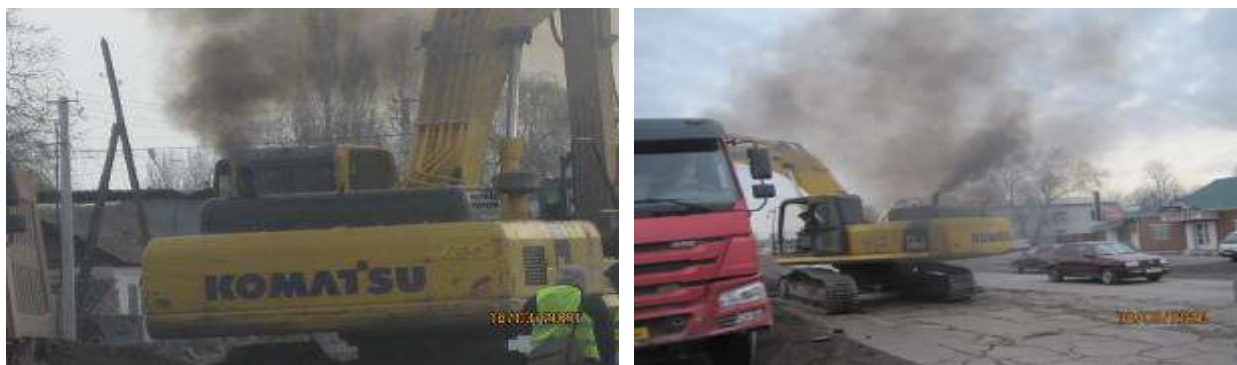
Figure 52 Unsatisfactory technical condition of the excavator
