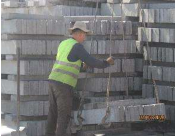
Figure 68 Safety violations when moving loads with a crane and working at height
