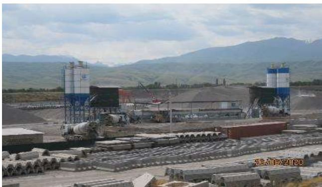
Figure 16 Concrete mixing plant
