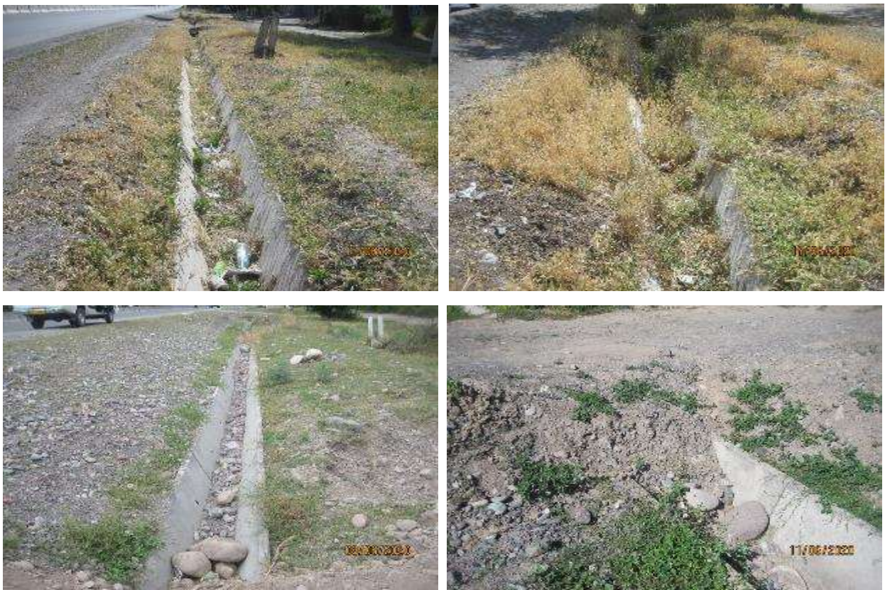
Figure 30 State of the previously installed chutes
