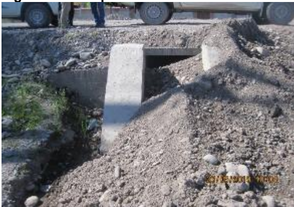
Figure 12. Newly built culvert blocked with construction debris.
