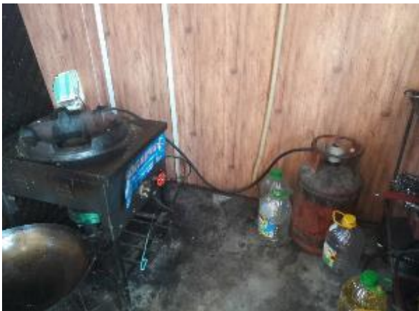
Figure 17. Placement of propane tanks near open flame
