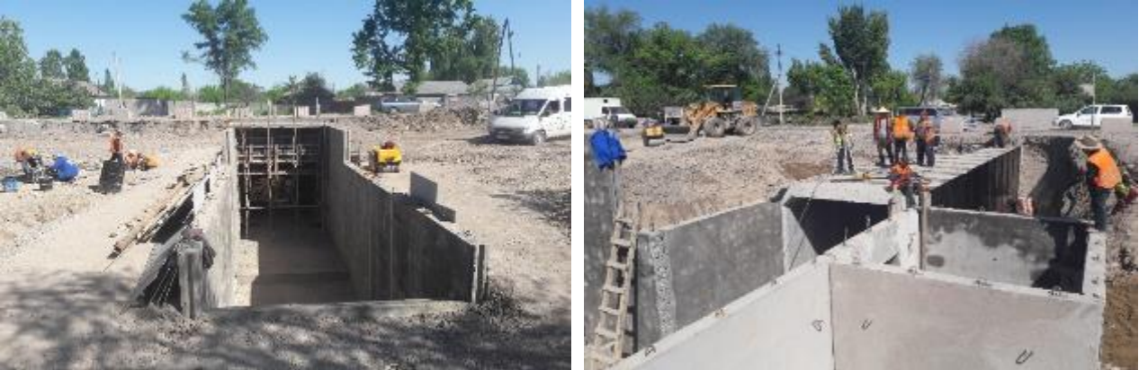
Figure 5. Underground pedestrian crossing and flooding issue
