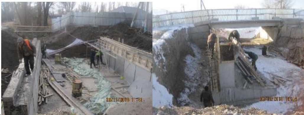
Figure 422. Carrying out of works at height without PPE
