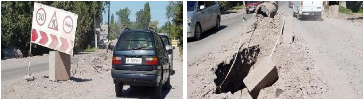
Figure 21. Dangerous construction practices, Belavodsk
