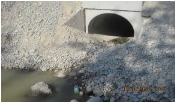
Figure 28. Debris almost totally blocking new culvert entrance
