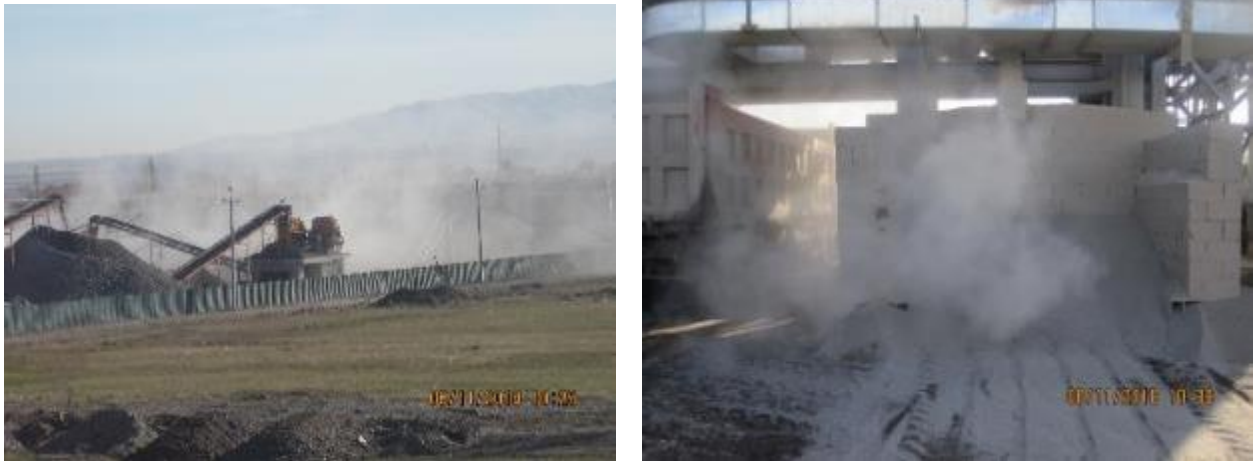
Figure 398. Dust in the aggregate processing plant and the asphalt plant
