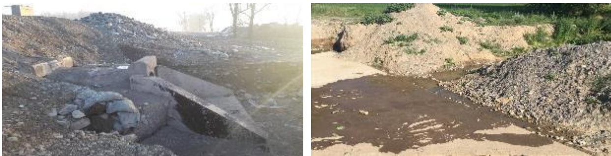
Figure 29. The culvert with an extra section added and Jelamysh R. bridge blockage
