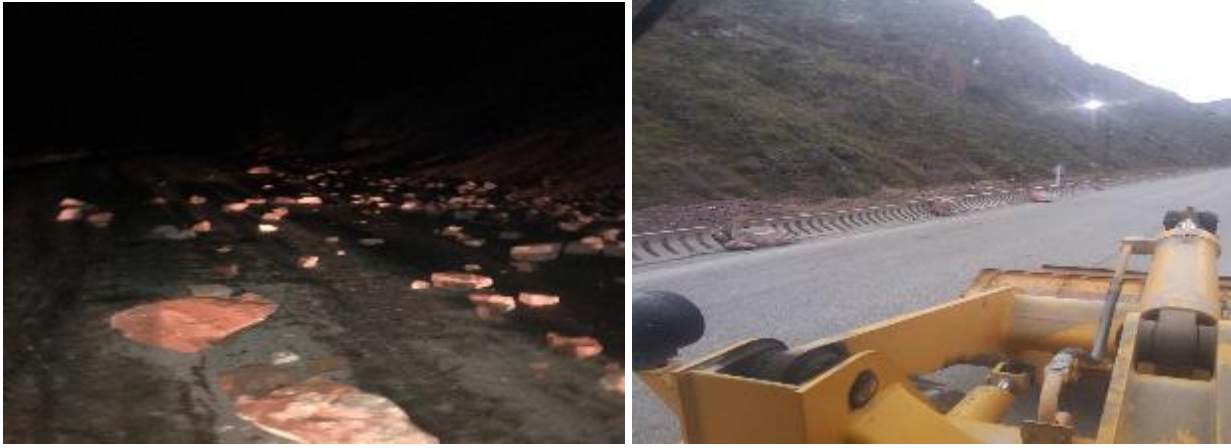
Figure 11. Danger of rockfalls
