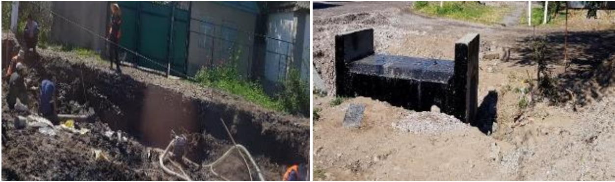
Figure 20. Unsafe Construction Practices, Alexandrovka Village
