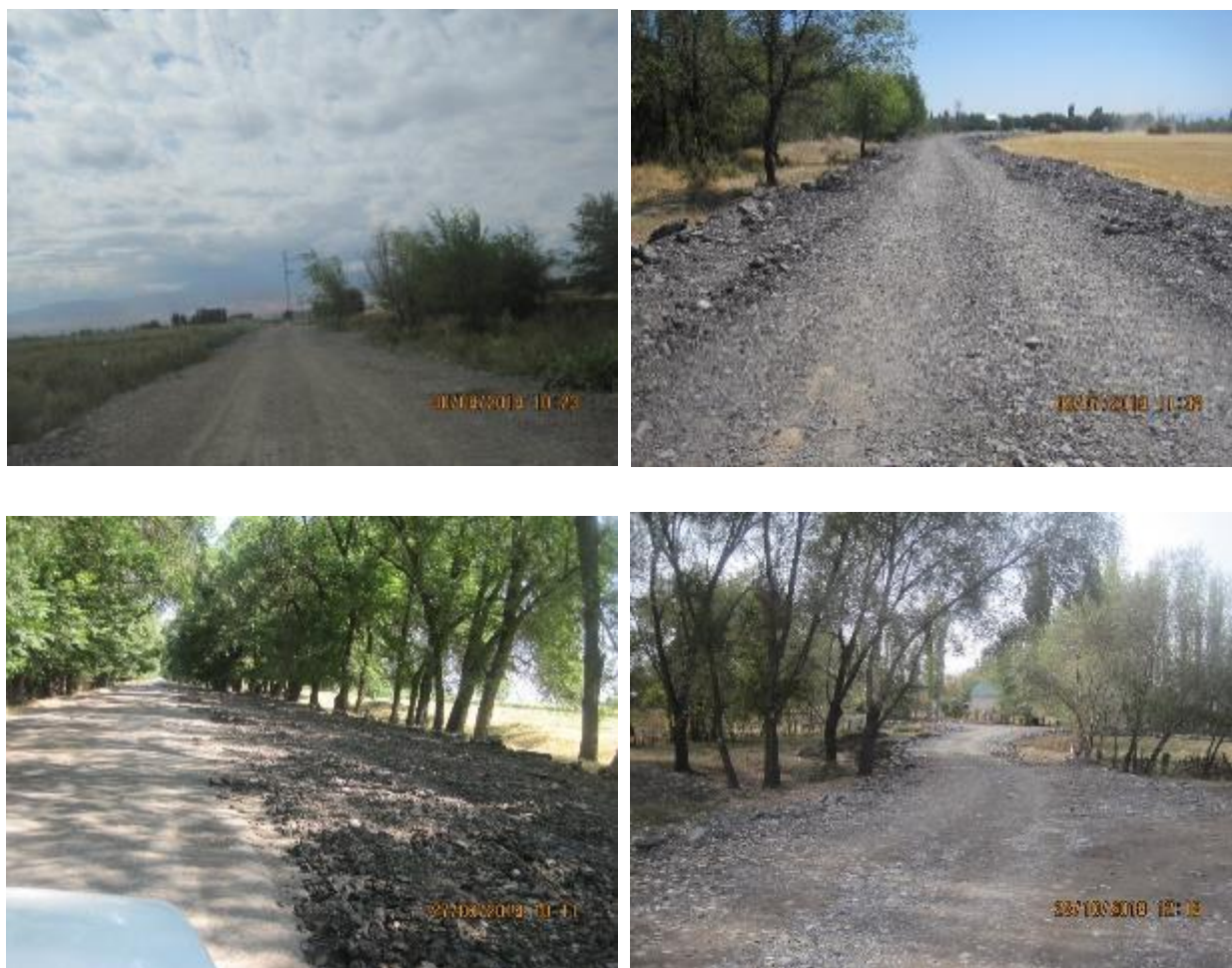
Figure 400. Old asphalt on local small roads and laneways
