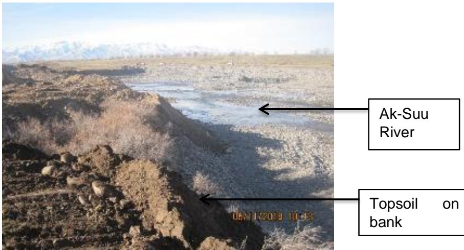
Figure 311. Topsoil incorrectly stored at the river shore
