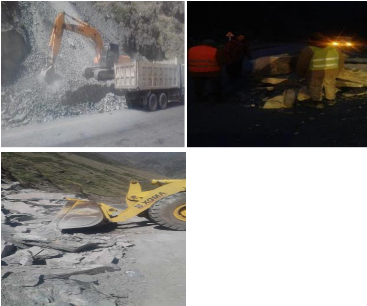
Figure -8. Rockfall hazard
