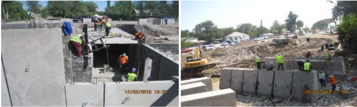
Figure 68 Working at height without personal protective equipment
