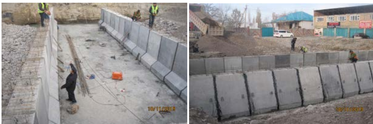
Figure 37 Safety violations during the construction of the bridge at the Jantai canal
