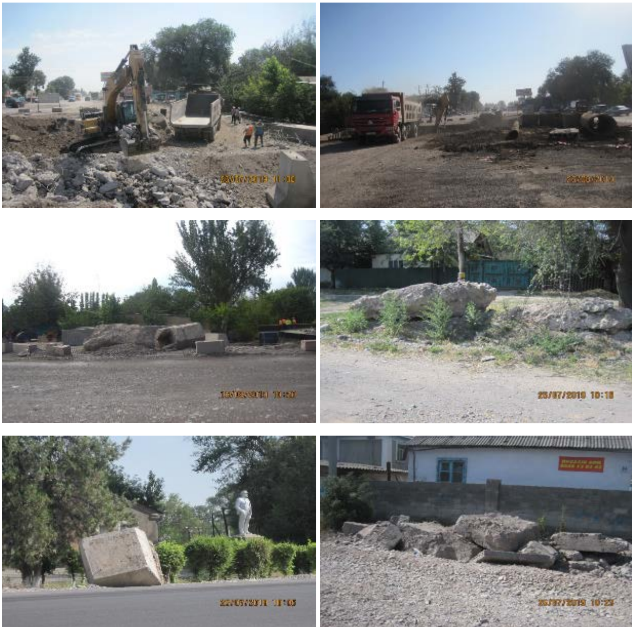
Figure 48 Construction waste on the road
