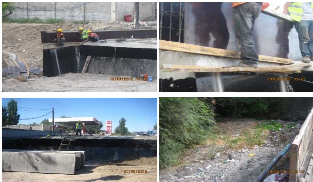
Figure 35 Safety violations during the construction of the bridge at the Krepostnoy canal
