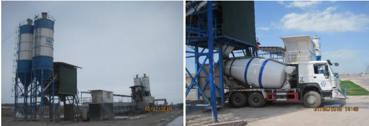
Figure 18 Concrete mixing plant
