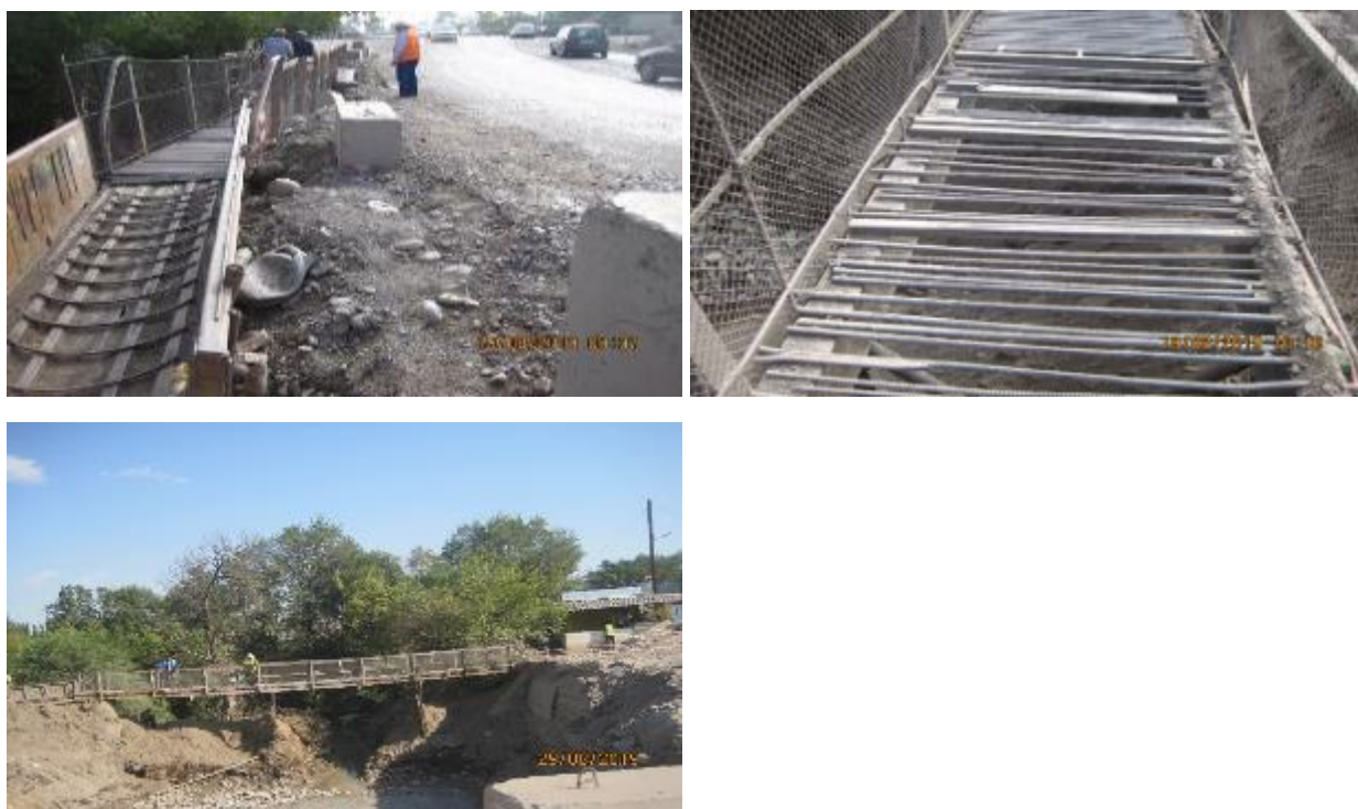
Figure 34 Violations during the construction of a pedestrian bridge at the Krepostnoy canal
