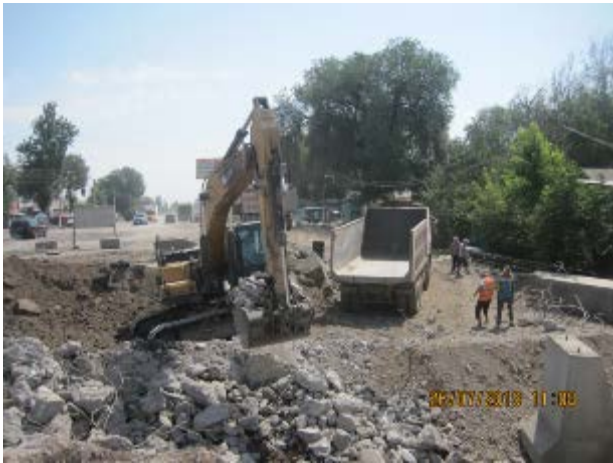
Figure 31 Waste accumulated during the construction of the bridge
