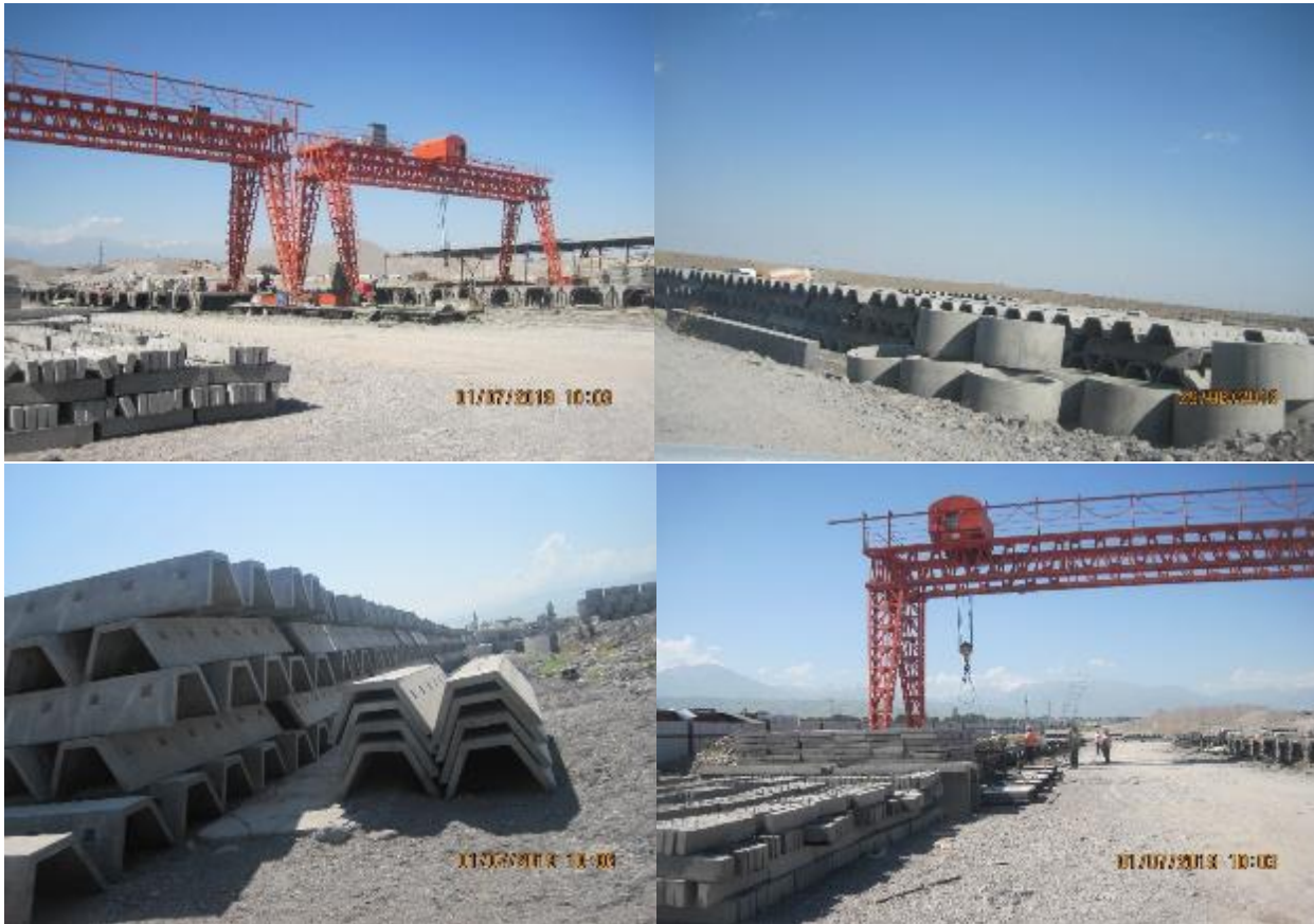
Figure 19 Polygon for production of reinforced concrete products
