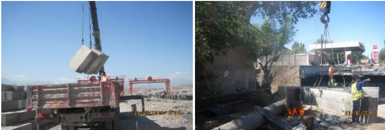
Figure 69 Safety violations when crane operates
