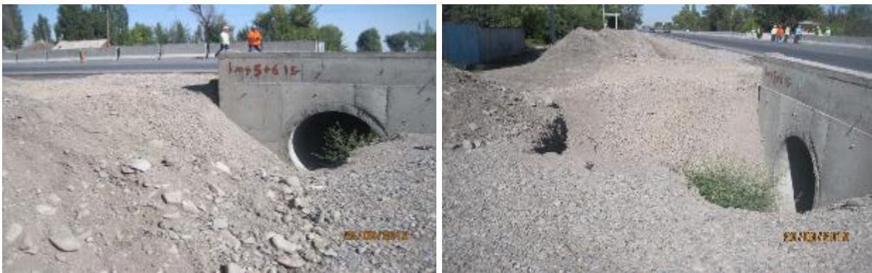
Figure 28 Violations on the constructed structures
