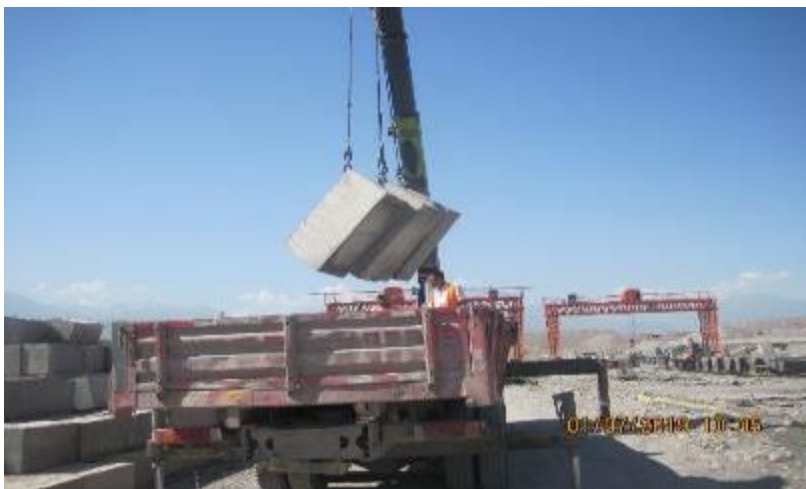
Figure 46 Violations of safety precautions at the site of production of reinforced concrete structures
