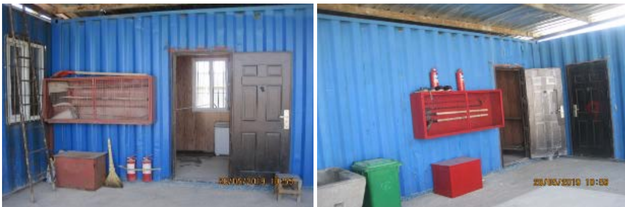
Figure 23 Fireshield equipment at the camp
