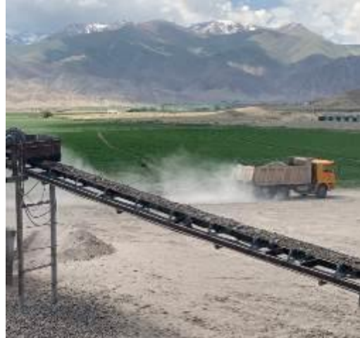
Photo 69. Lot 2. Lack of watering earthen roads.
