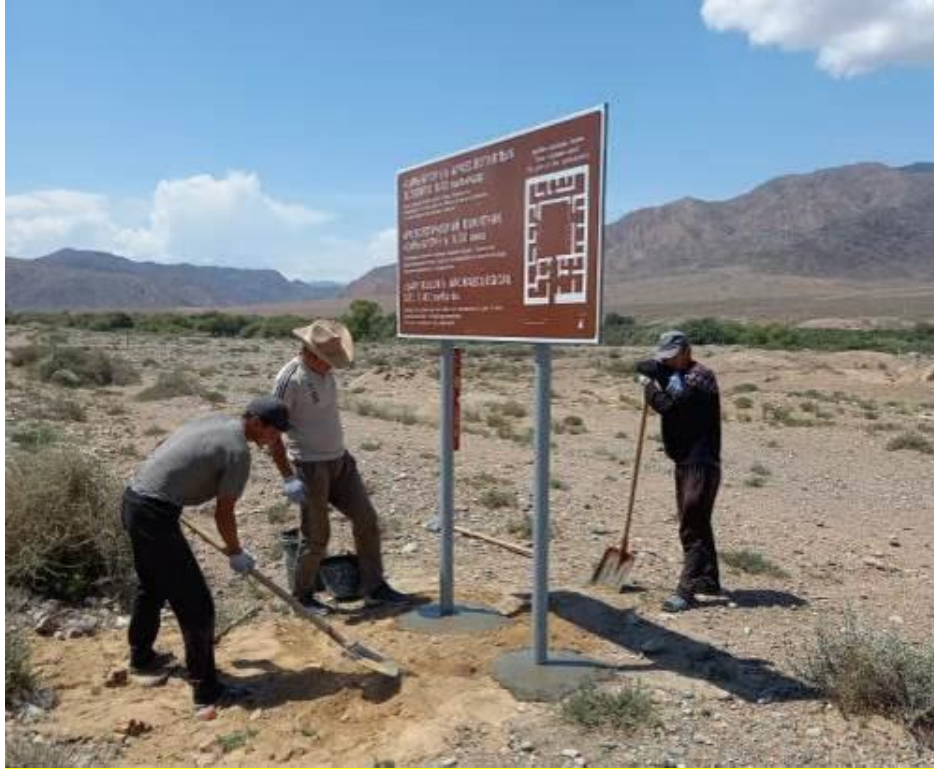
Photo 10. Installation of an information panel on the Archaeological Monument "Sary-Bulun I" X-XII centuries. Iron ore processing workshop. Km 7 + 300 RHS of the road.
