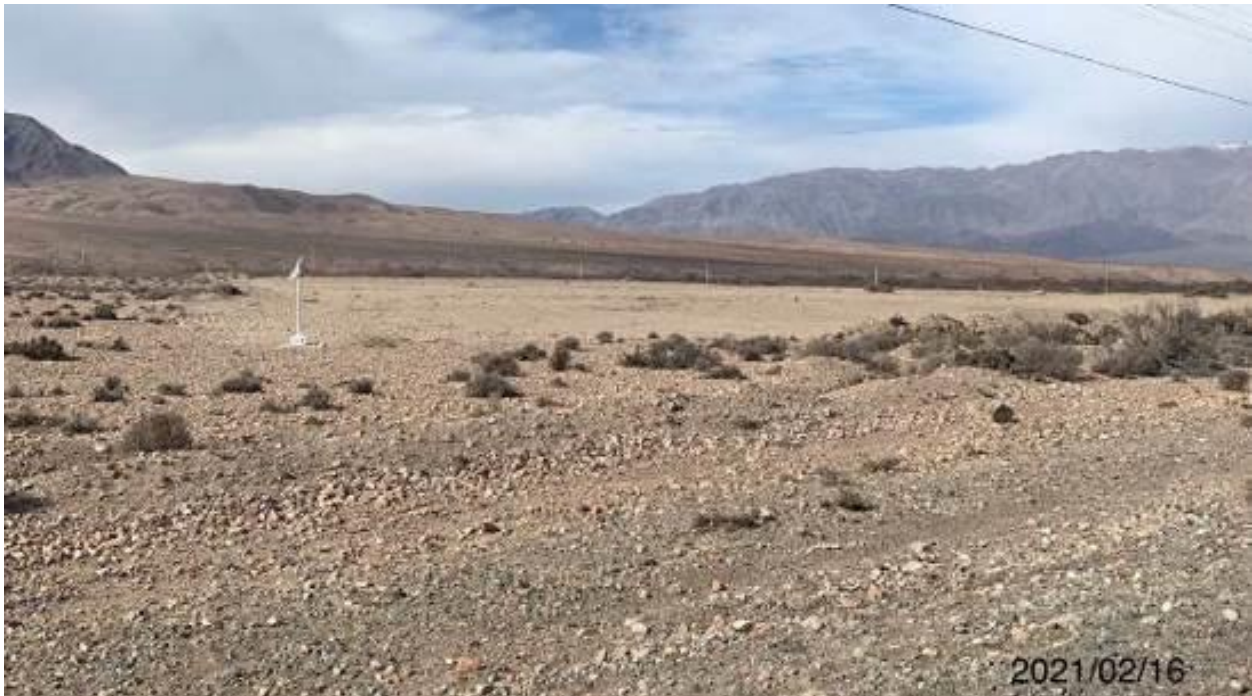
Photo 105. Lot 1. Quarry km. 9 + 000. The soil and vegetation layer were removed, and the boundaries of the quarry territory were marked by installing white racks with flags.
