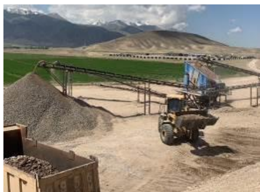
Photo 72. Lot 2. Work of crusher plant after the installation of the irrigation system with water: no dust.
