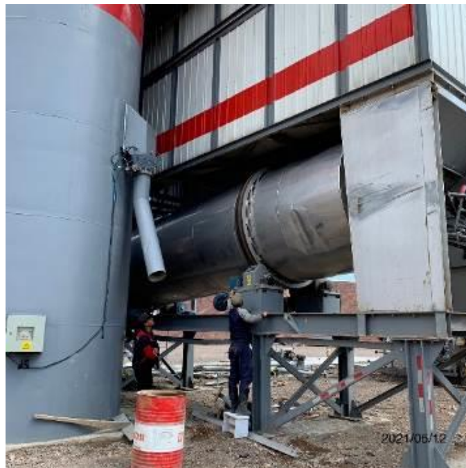
Photo 56. Concrete plant worker with no personal protective equipment.
