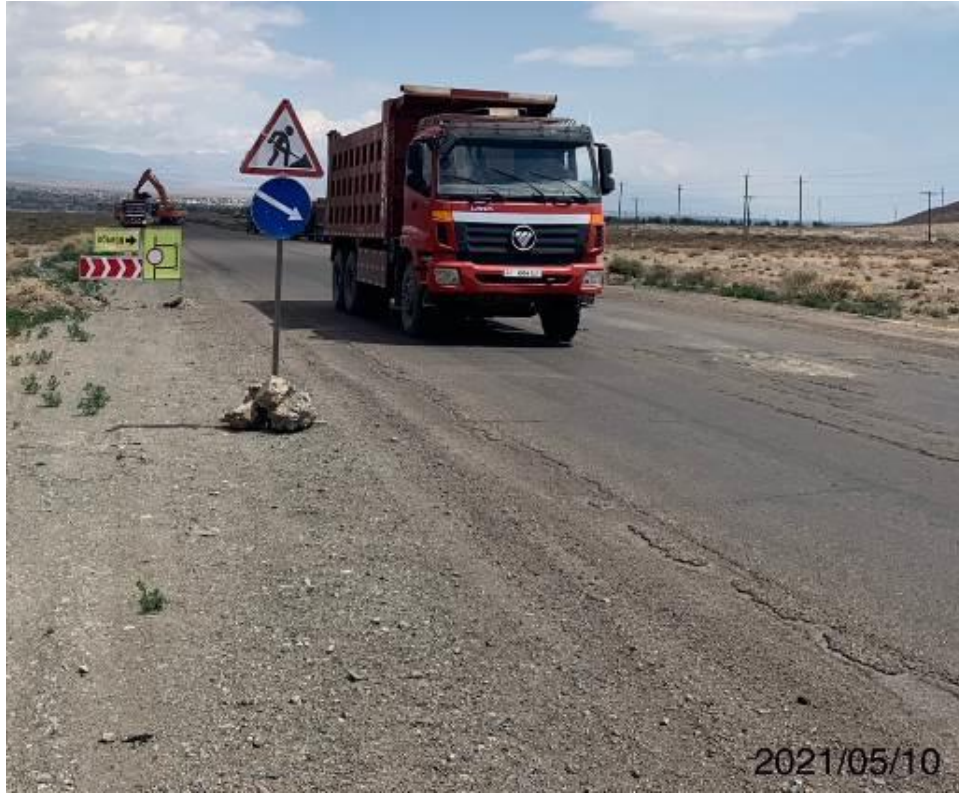
Photo 21. Lot 1. Warning road safety signs at km 4 + 800.
