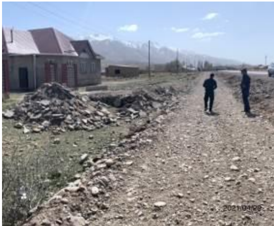
Photo 83. Violated passage to the house.
