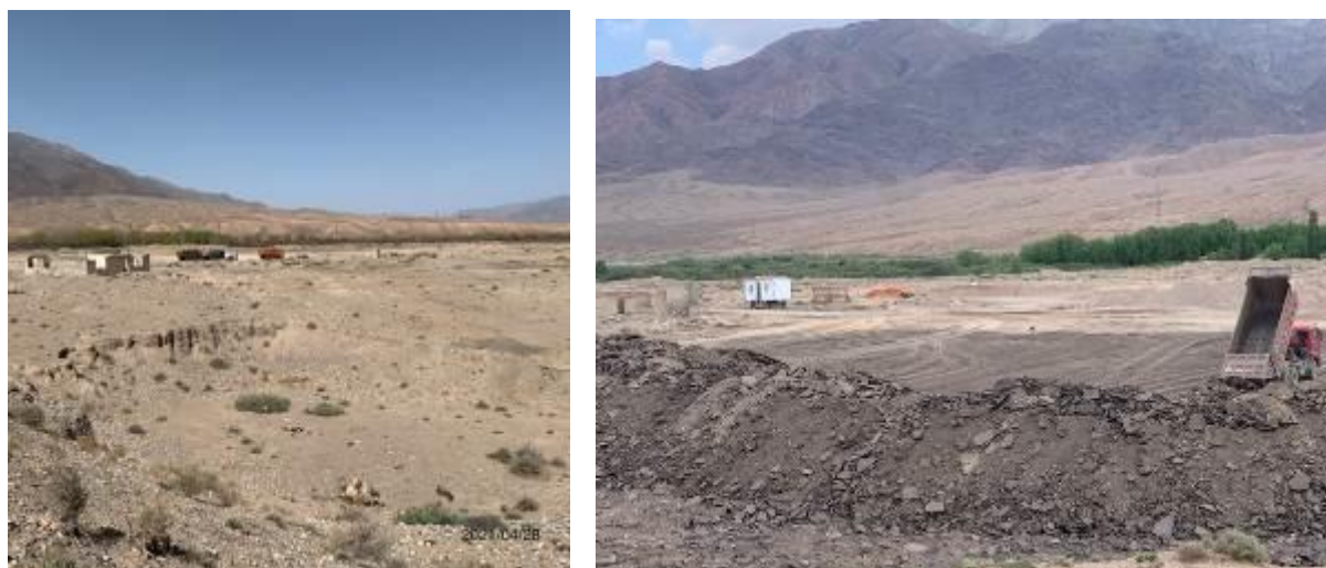
Photo 82. Spoil bank of old asphalt concrete at km. 7 + 100LHS before disposal, on the right during disposal.
