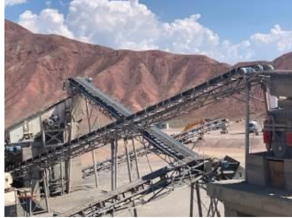
Photo 100. Lot 1. During the operation of crusher plant, dust emission is observed. Hydraulic irrigation system provided at crusher plant.
