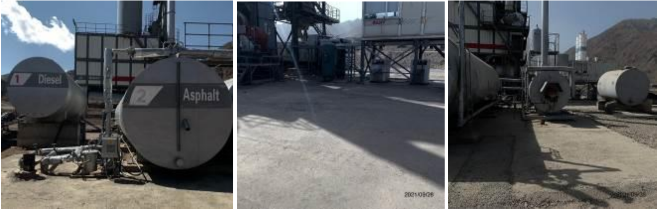
Photo 56, 57, 58 Provided asphaltting and concreting of production site and warehouses of fuel and bitumen at asphalt plant.
