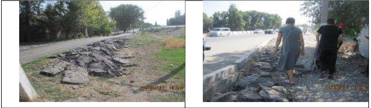
Figure 43. Asphalt scraps on the road.
