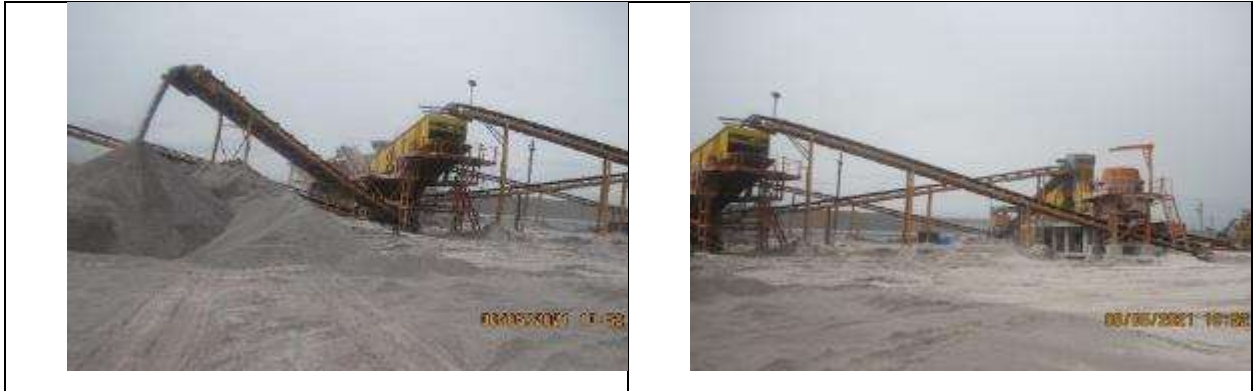
Figure 34 Stone crushing plant.
