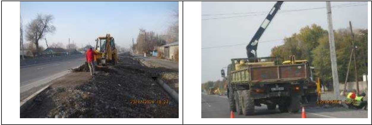
Figure 18 Preparation of pits and installation of lighting poles on the project road.
