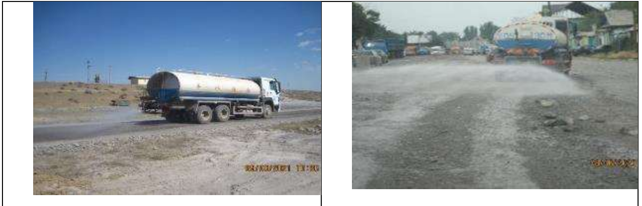
Figure 41 . Water sprinkling works. The road to the Ak-Suu 2 borrow pit and the road construction site in the village of Sokuluk.
