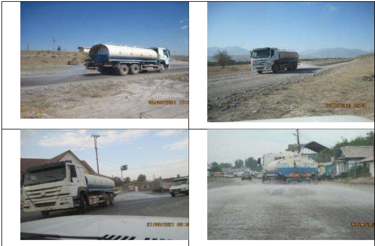
Figure 23 Water sprinkling works. Road to the Ak- Suu 2 borrow pit and at the construction site in the Sokuluk village.
