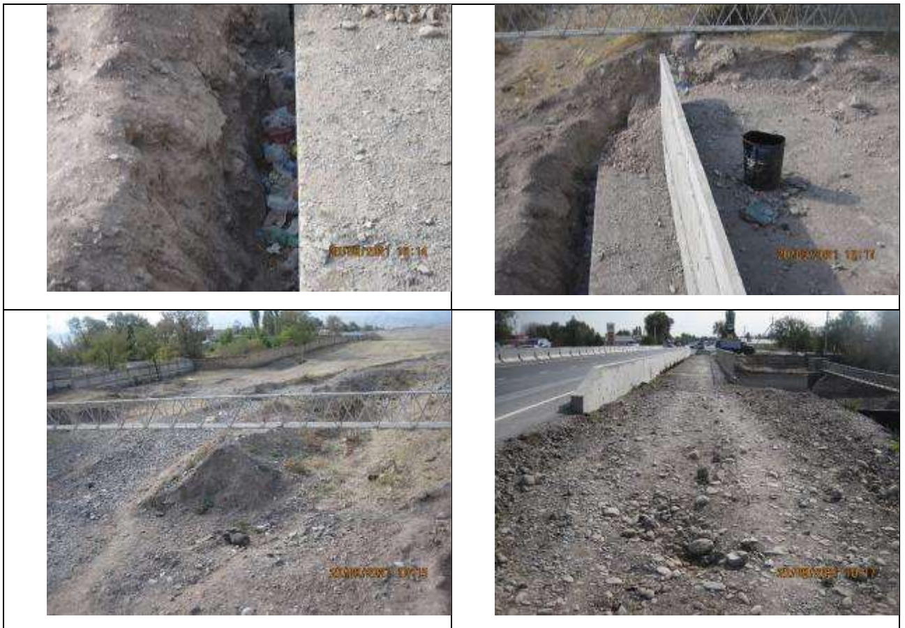
Figure 46. Ak-Suu River after unfinished construction.
