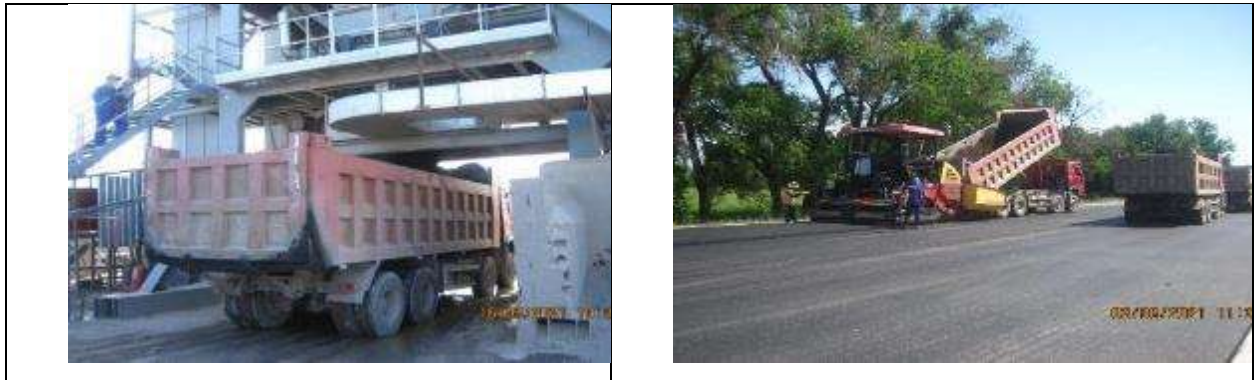
Figure 37 Loading of asphalt mixture into dump trucks and unloading into asphalt pavers.
