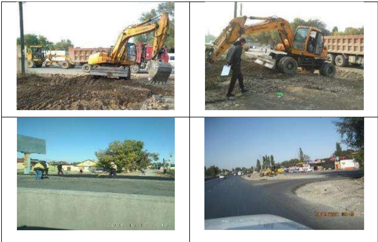
Figure 7 Laying asphalt at the junctions to the streets adjacent to the road in the Alexandrovka village.
