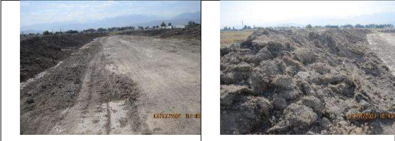
Figure 92. An area for storing unsuitable soil after removing the top layer. Stored soil.
