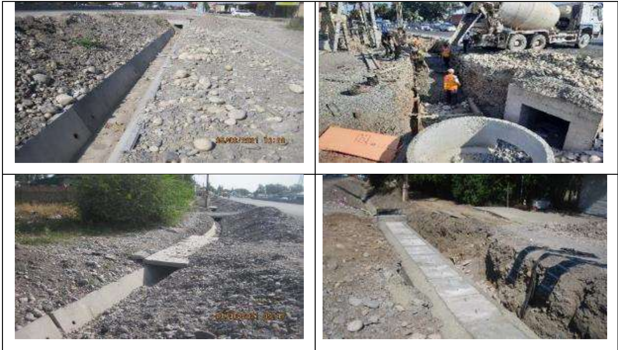
Figure 10 Installation of roadside ditches and crossings to private houses and streets adjacent to the road in the Alexandrovka village.
