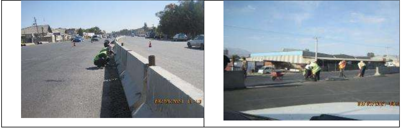
Figure 42. Works on concreting of ditches on the carriage way between the parapets.
