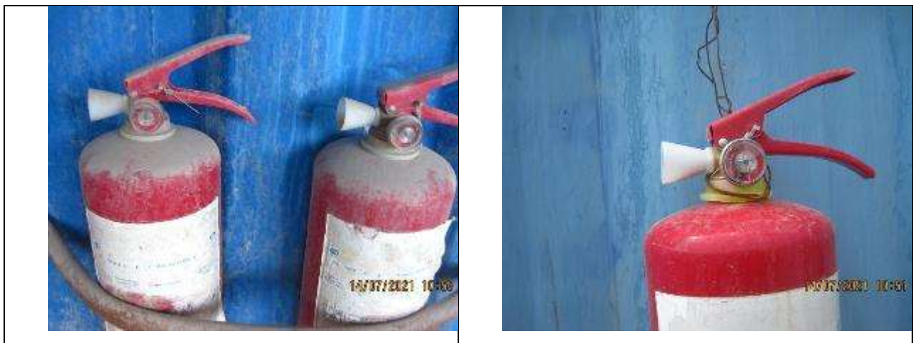
Figure 66 Fire extinguishers installed with violations on the territory of the production site.
