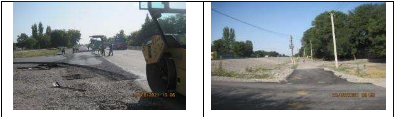
Figure 8 Laying asphalt at the junctions to the streets adjacent to the road in the Petrovka village.
