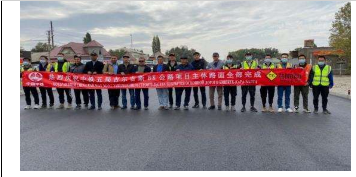
Figure 6 Completion of asphalt pavement works on the main road from km 15.9 to km 61.
