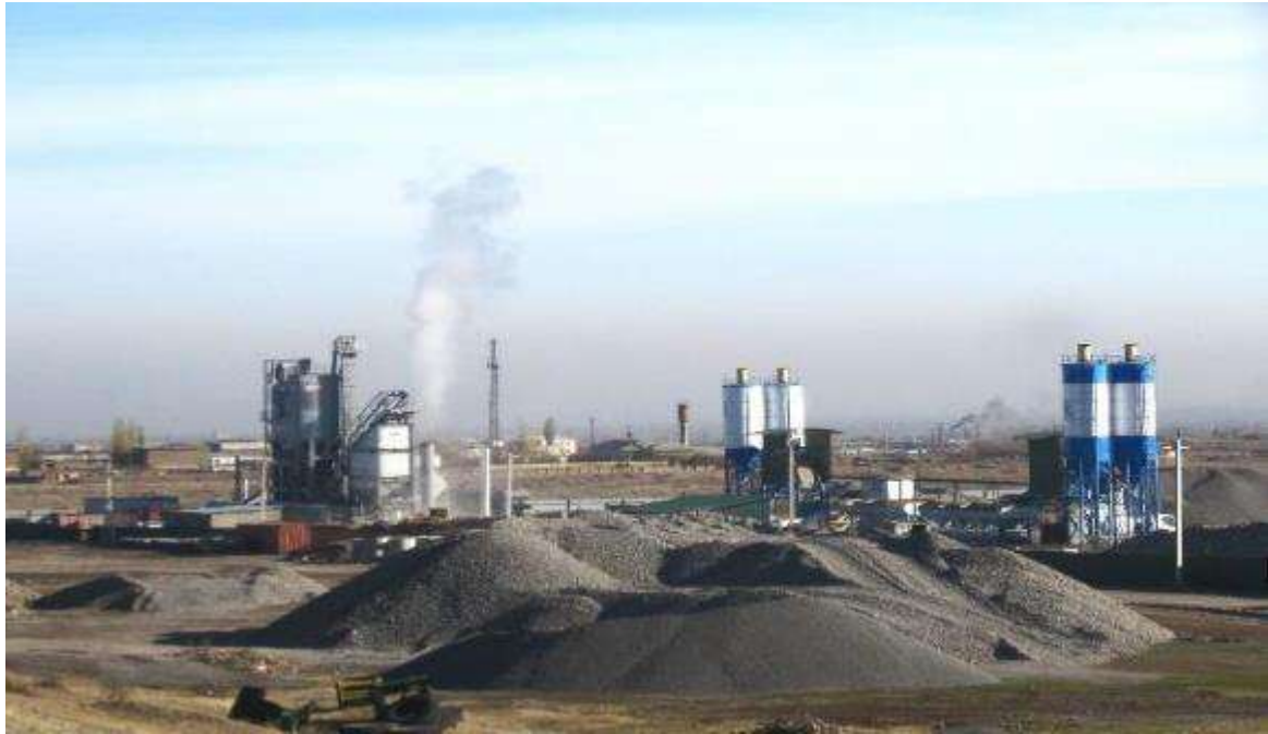
Figure 32 Production site. Concrete mixing plant. Asphalt Concrete Plant
