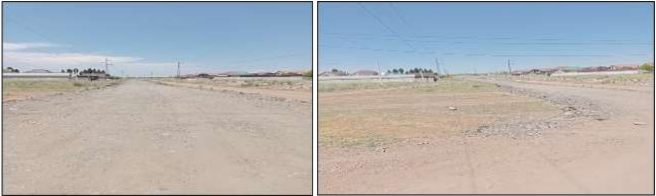
Figure 71 Removal of old asphalt to the territory of the "Altyn Ordo" residential area at the request of residents and representatives of local government
