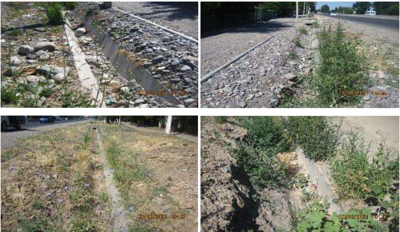
Figure 34 Condition of previously installed chutes
