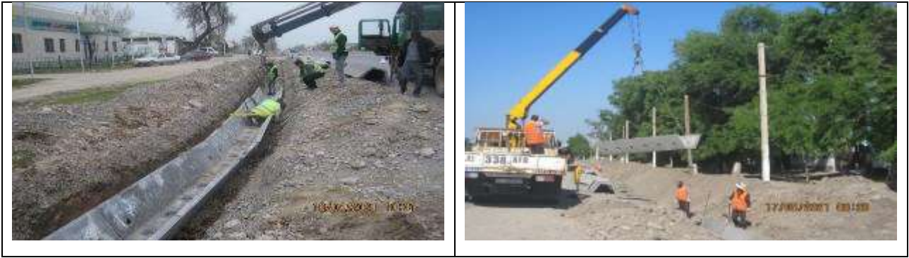
Figure 33 Violation of safety precautions during installation of culvert chutes.
