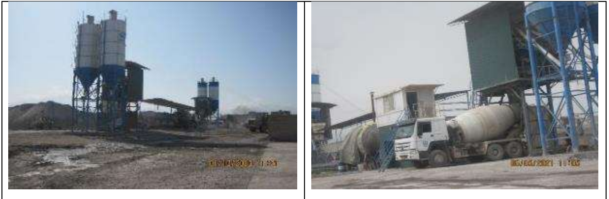
Figure 23 Concrete mixing plant
