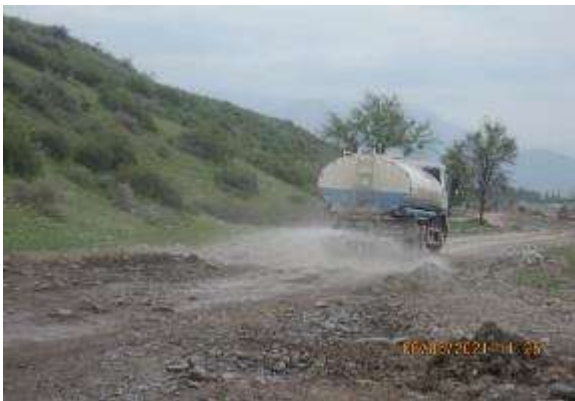
Figure 16 Water sprinkling on the road to Ak-Suu 2 borrow pit to avoid dusting
