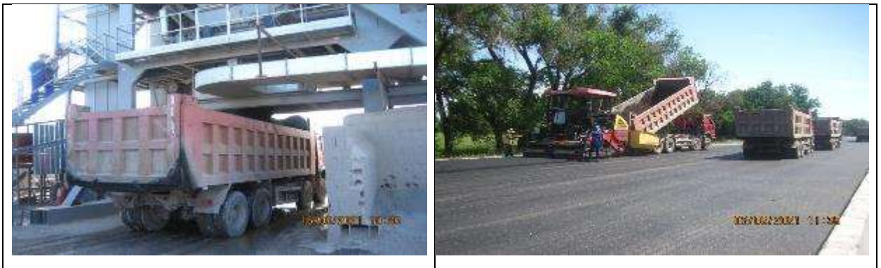
Figure 24 Loading of asphalt mixture into dump trucks and unloading into asphalt pavers
