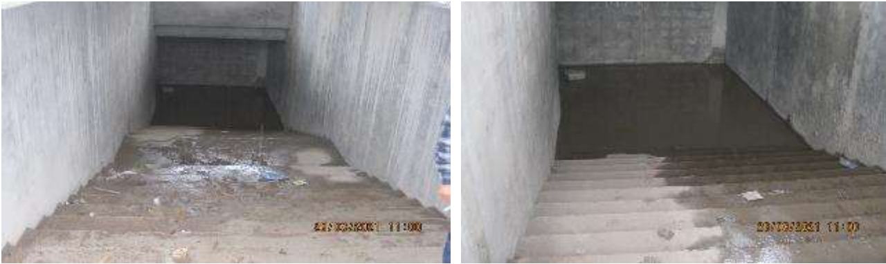
Figure 39 Underground passage flooding at km 57 + 420 during the rainy season in March 2021
