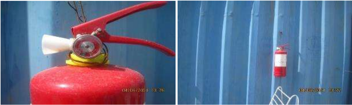
Figure 54 Fire extinguishers installed with violations on the territory of the production site
