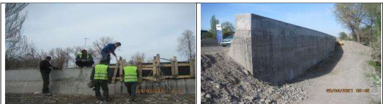
Figure 38 Violation of safety precautions when working at height
