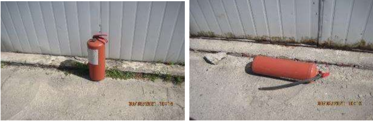
Figure 56 Fire extinguishers installed with violations on the territory of the base in Sokuluk
