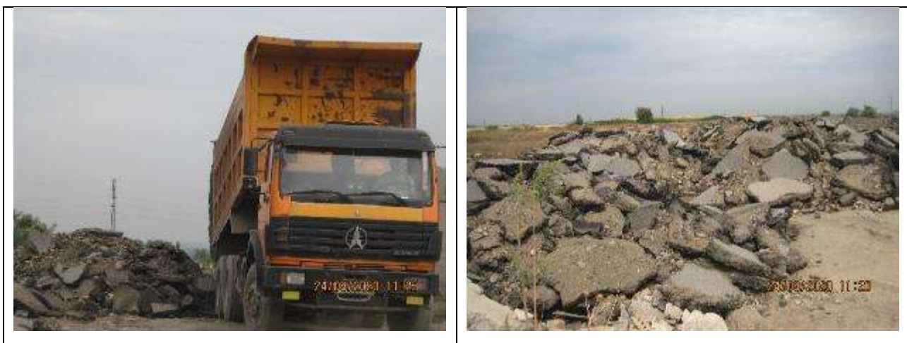
Figure 70 Dumping of old asphalt on designated sites for further use in the Romanovka
