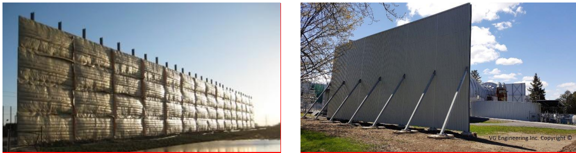
Figure 5.1: Examples of Temporary Noise Barriers
