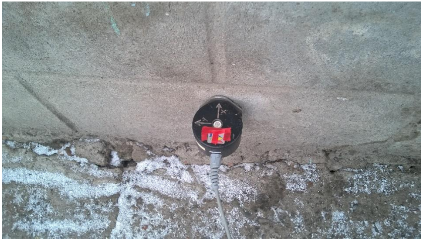
Figure 1. Location of Geophone on Foundation of Building
