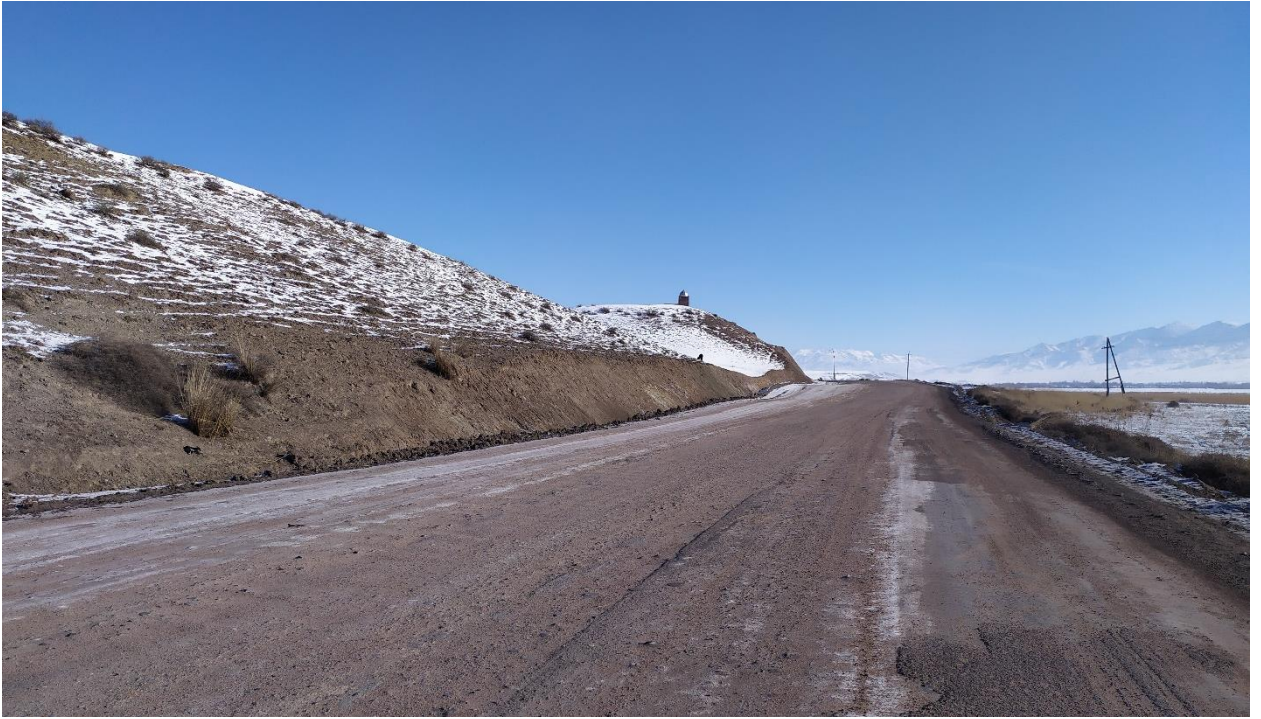
Fig. 31. Tugol-Sai 1-2-3. Road construction process. A hill with mounds at the top is LHS.
