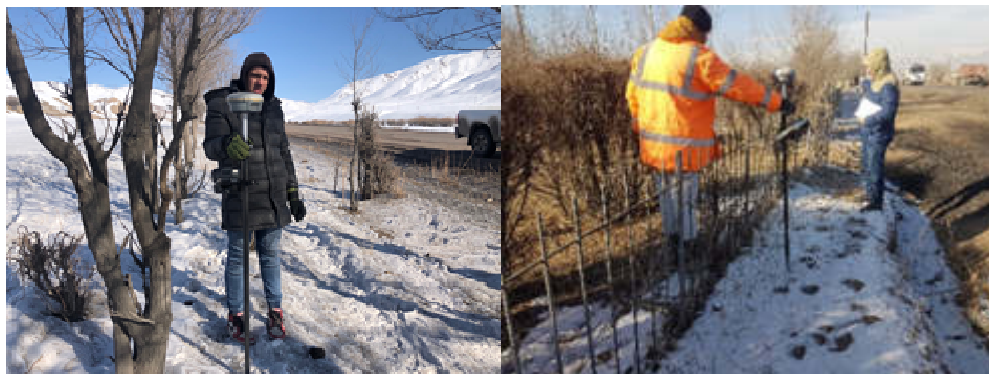
Clarification of objects and AP's, work with engineers, representatives of local authorities and Gosregister
